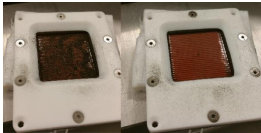
Figure 4: Before and after clearing dust once the HVPS connection was fixed.
