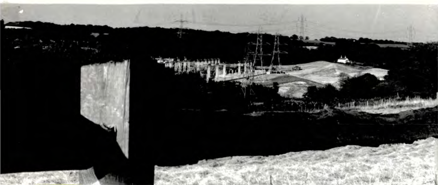
Photograph 40. Ninfield substation is regarded by the Board as one of the best examples of good siting from an amenity point of view. The substation structures that were coloured grey are barely distinguishable in the top left of the photograph.
