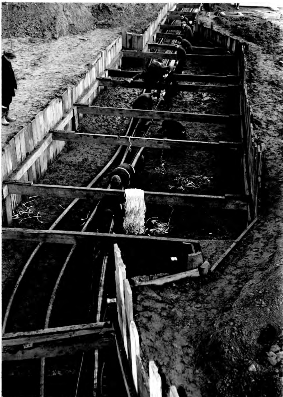
Photograph 29. Shows the width required to join the three phases of one 400 kV cable circuit.
