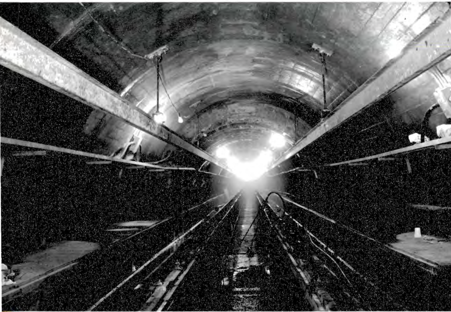
Photograph 33. Southampton Water cable tunnel before installation of cables.
