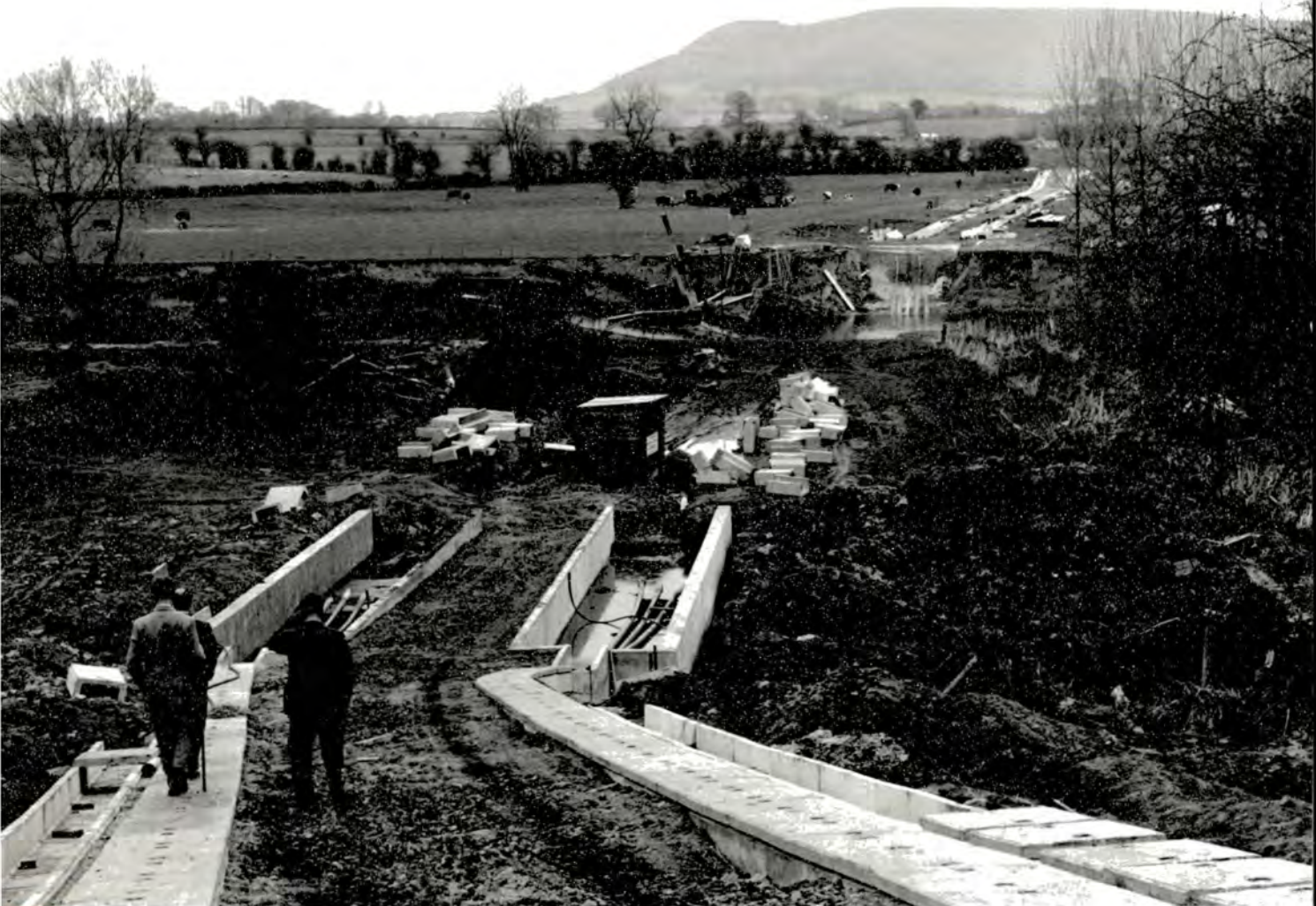
Photograph 35. Installation of concrete troughs for 400 kV cables at approach to the River Wye.
