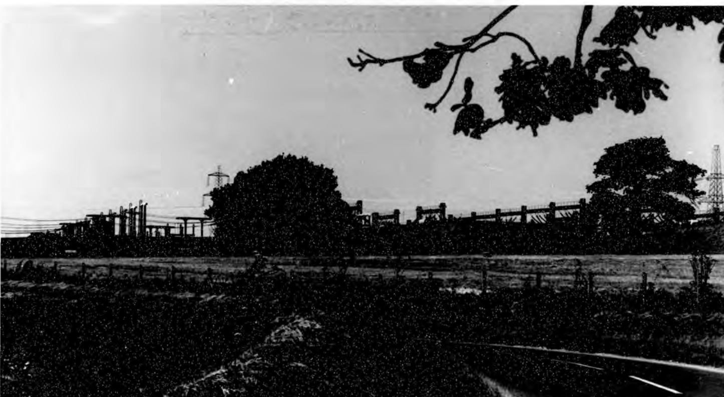
Photograph 78. Lovedean substation, taken in October 1966, soon after the completion of the ground modelling.
