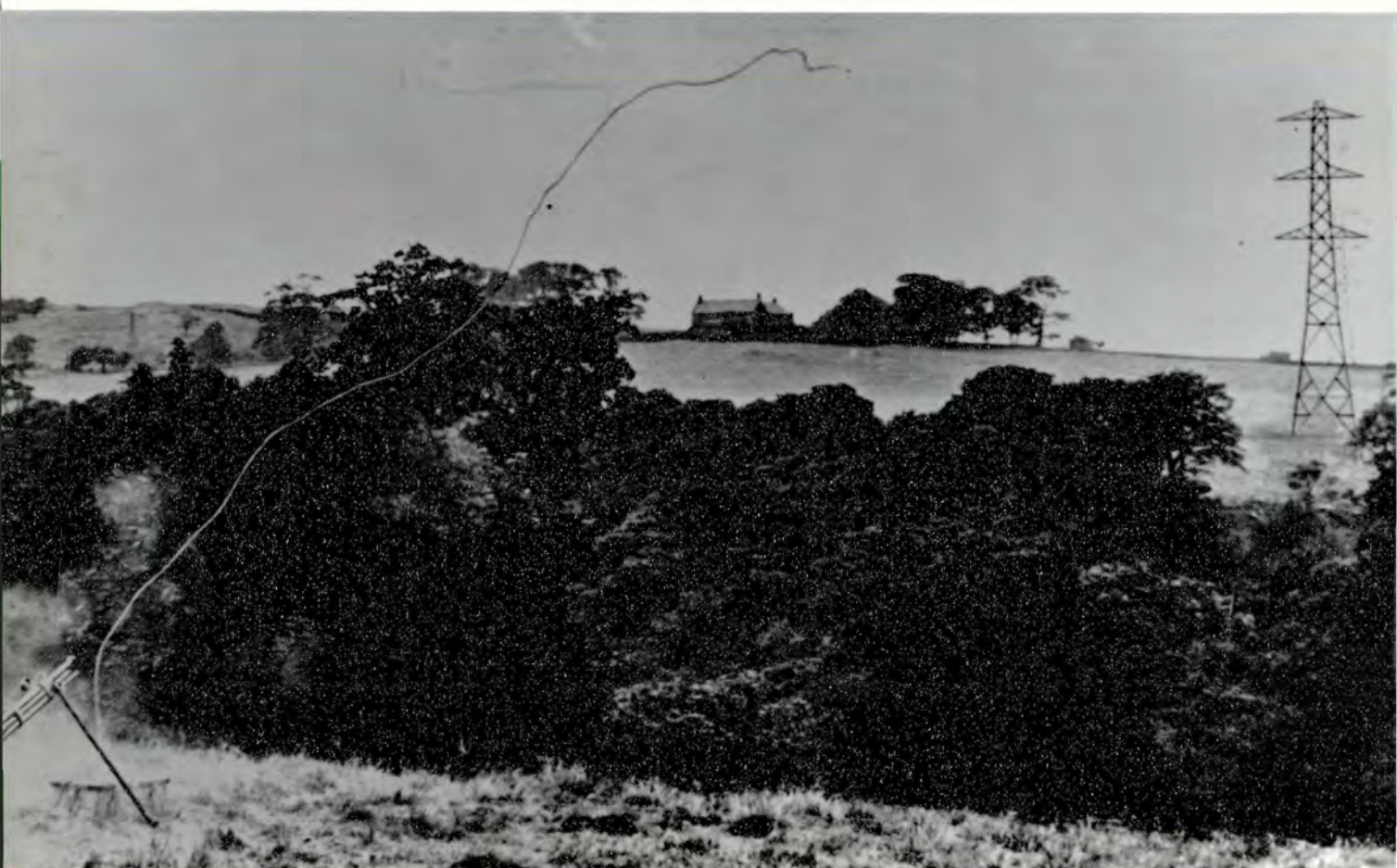
Photograph 23. A rocket carrying a pilot line was used to span the Nant y Ffrith valley, so that conductors could be pulled across without the need to fell the trees.
