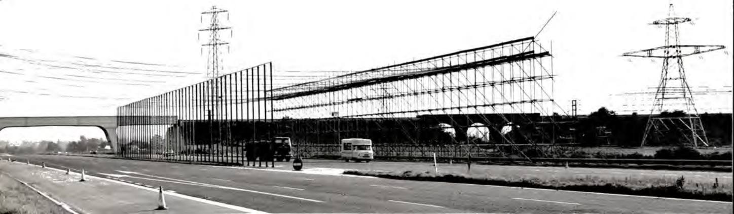
Photograph 6. Showing the extensive scaffolding required to support conductors during construction across the M.4 motorway.
