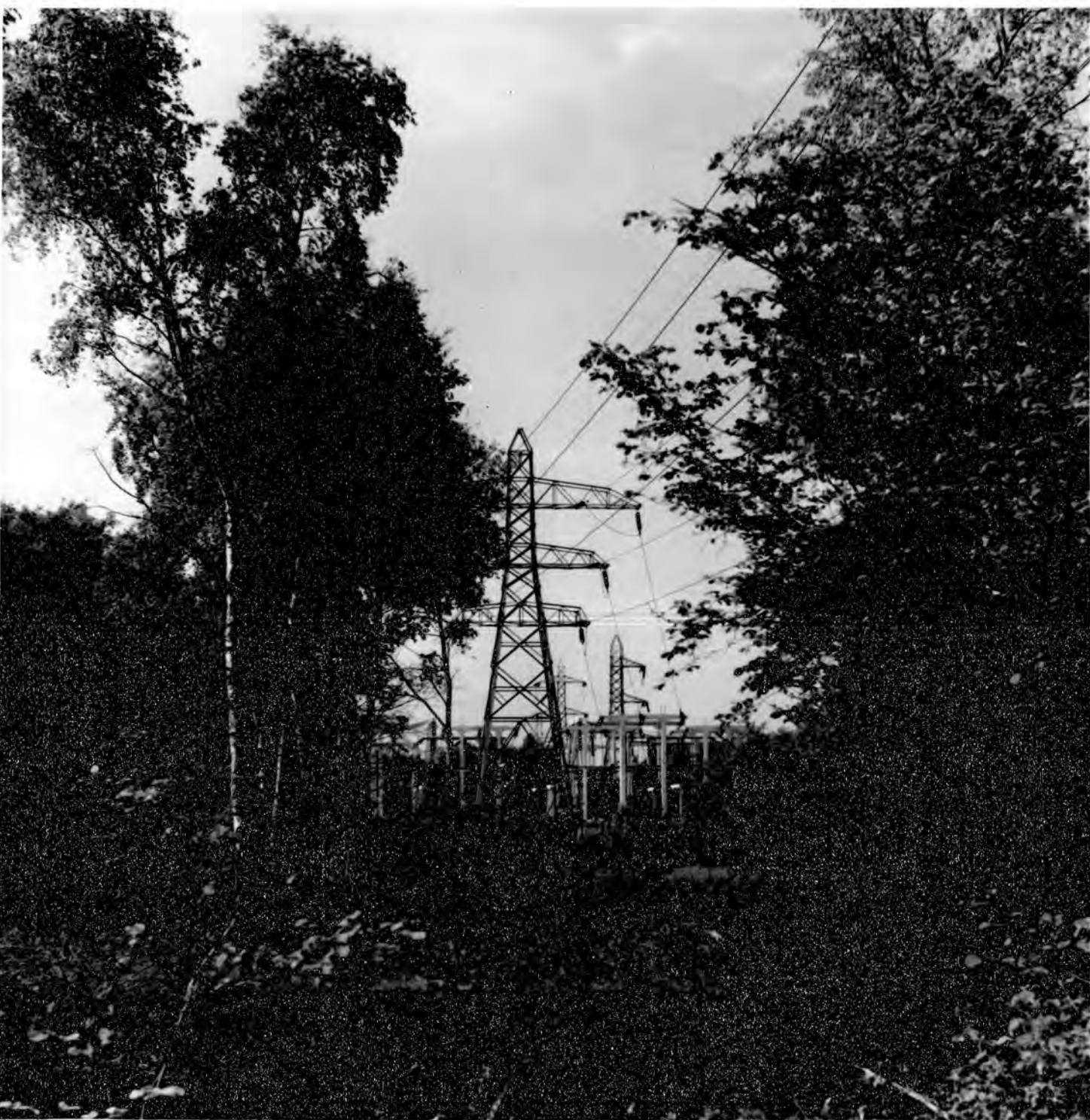
Photograph 49. The siting of Fleet substation in Coxmoor Wood has provided complete and effective screening from all public viewpoints. This view was taken within the wood in a small area cleared to permit erection of the overhead line.
