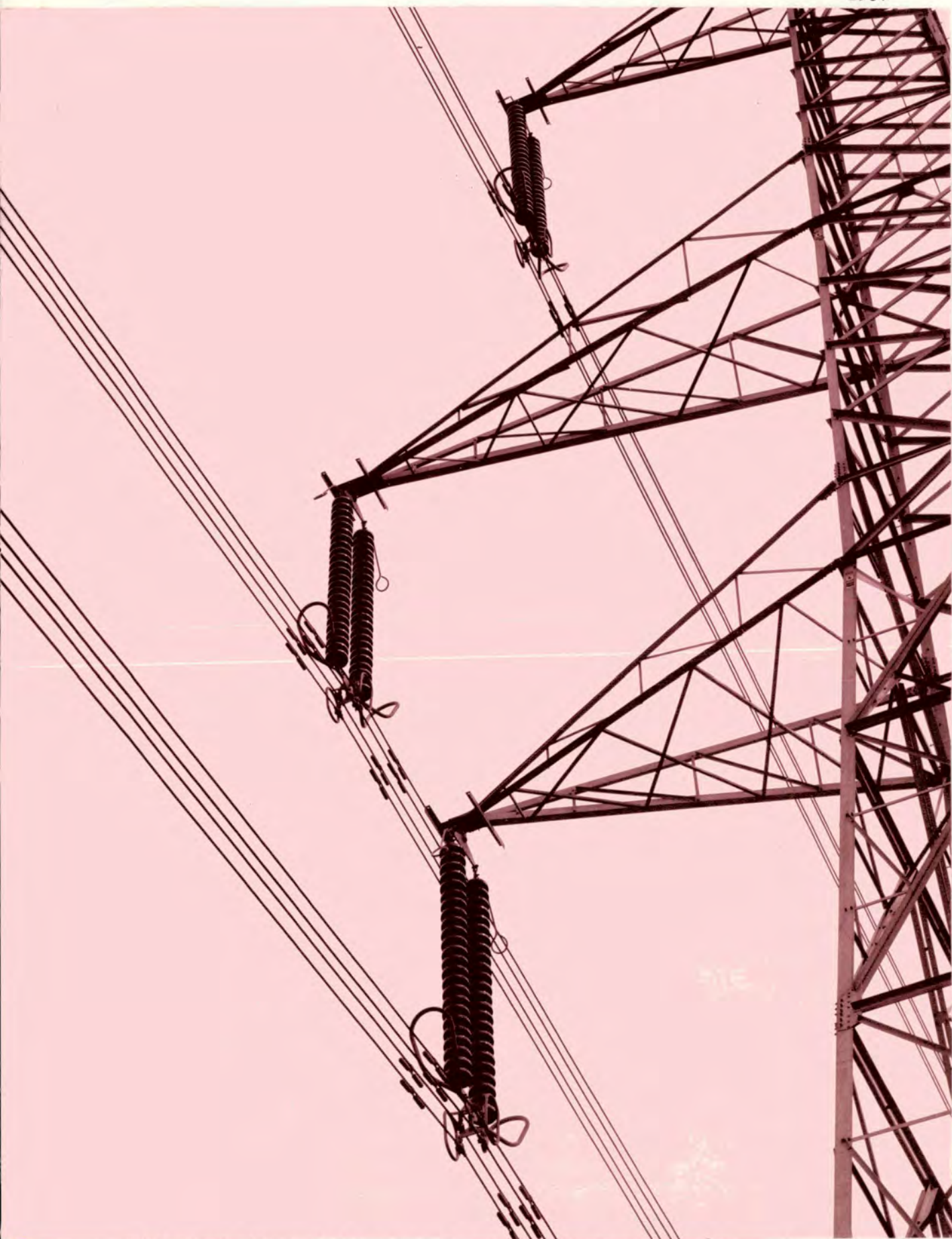
Photograph 63. A 400kV suspension tower showing two strings of porcelain insulators to carry a bundle of four conductors.
