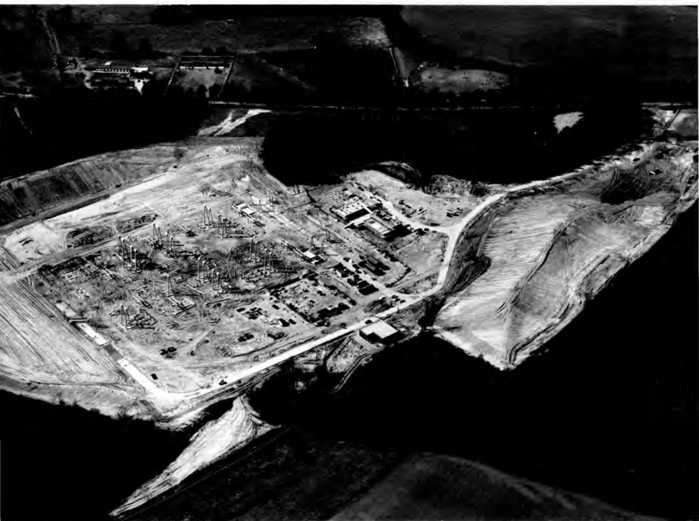
Photograph 76. Air oblique view of Hurst 275/132 kV substation looking westwards. London Borough of Bexley. M.R.489730. This photograph taken on Wednesday, 9th April 1969 shows the substantial completion of the preliminary earthworks just prior to grass seeding. This site is generally regarded as being a very good one from a visual amenity point of view as the substation has been carefully located between Sands Spinney to the top right of the photograph, Cavey's Spring in the bottom right, and a Forestry Commission Plantation on the left. The only vulnerable aspect was to the east of the site where land modelling 40 ft. high has been carefully designed and shaped to provide a line of visual cut off for the occupants of dwellings further to the east. Planning permission required a landscaping scheme of which the ground modelling formed the first stage. The second stage tree planting will be carried out next year in order to clothe the new land form, and to complete the screening of the whole site. The care taken in site selection and landscaping will help to ensure that when the substation is finished it is unlikely that any of the local residents will even be aware of the existence of this major switching and transforming station in their neighbourhood.
