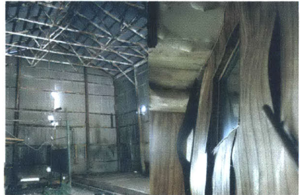
Site buildings beyond repair, July 2002
