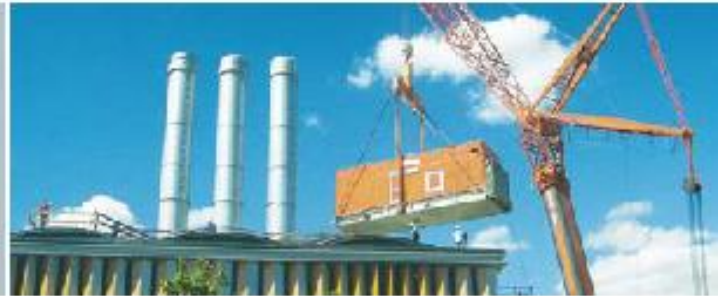
Rooftop installation in a cultural urban environment at Würzburg, Germany.
