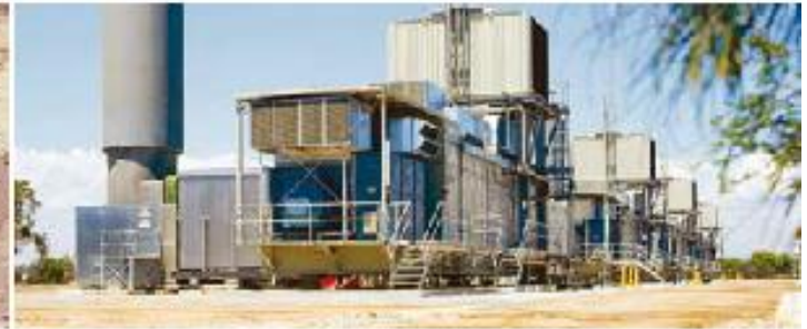
On Torrens Island, Australia, four SGT-600 gas turbines provide seasonal peaking support for the electrical grid.
