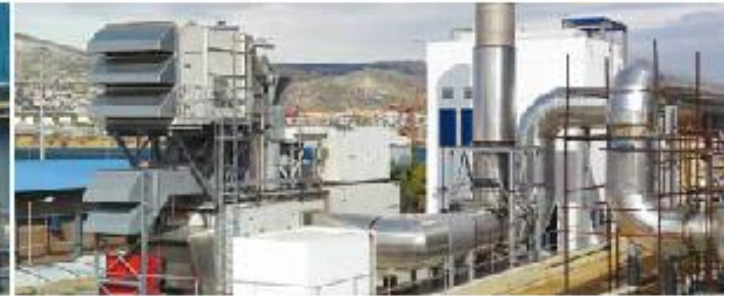
Sewage-sludge drying plant for the City of Athens, on Psyttalia island.
