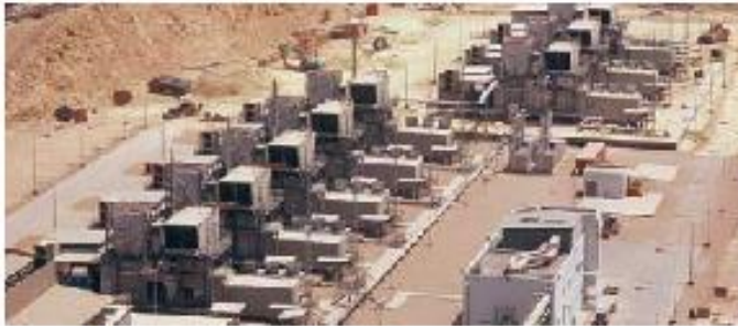
Two multi-unit deliveries of SGT-600 gas turbines power this cement factory near Riyadh, Saudi Arabia.
