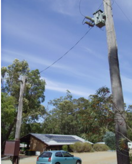
Figure 3.13: 10 kW transformer at the entrance of the monastery
