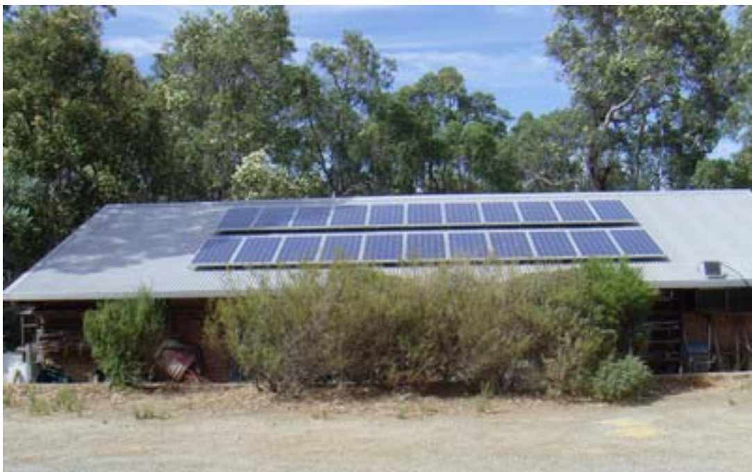
Figure 3.12: 22-190 W (4.18 kW) Solar PV system installed at the monastery
