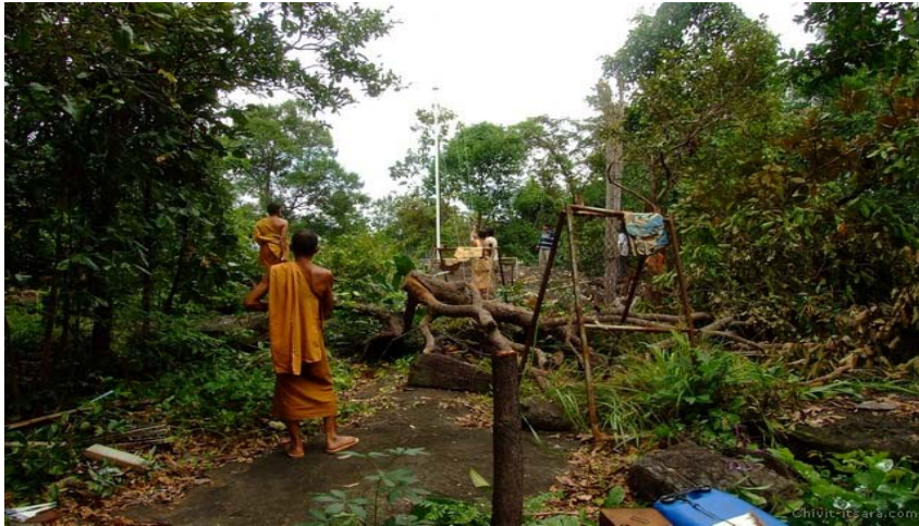
Figure 2.7 : Buddhist monks are watching the wind turbine installation at Thai Forest Tradition Temple in Thailand (www.chivit-itsara.com 2009)
