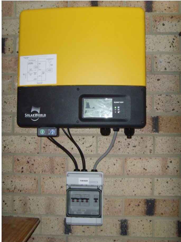
Figure 3.14: PV Inverter Sunny Boy 5000TL
