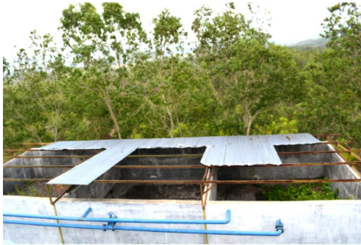
Figure 68. Current condition of slow sand filter in Kaligoro (Doc.: Marjianto, 2017)
