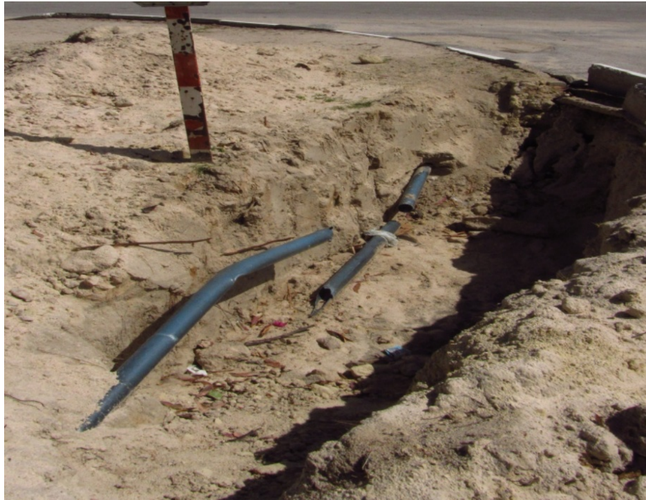
Figure 9. A damaged vacuum sewer in a trench in Old Ondangwa.
