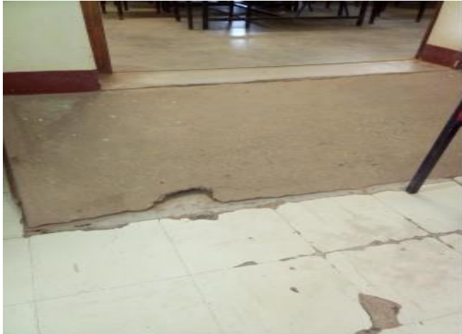
Figure 30: A floor with peeling tiles and chipping ramp in another library (Source: Field data, 2017)
