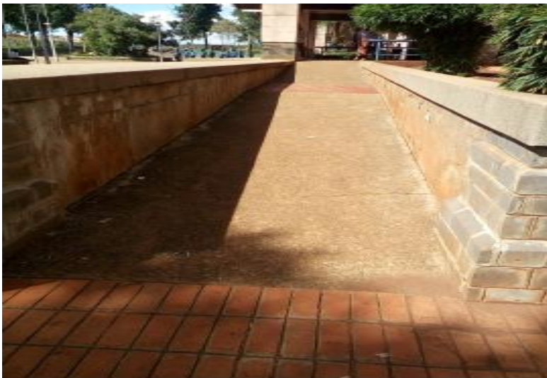
Figure 23: A ramp without hand rails at one of the libraries (Source: Field data, 2017)
