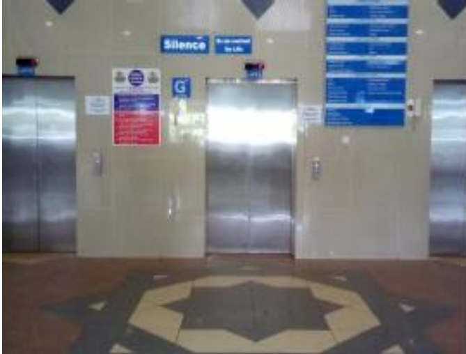
Figure 26: A set of lifts in one of the libraries (Source: Field data, 2017)
