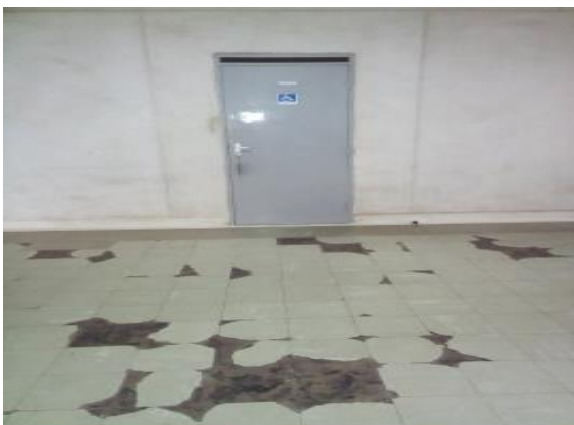
Figure 29: A floor with peeling tiles in one of the libraries (Source: Field data, 2017)
