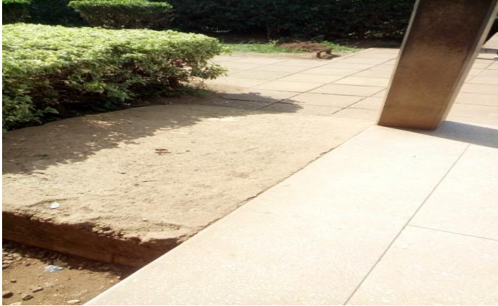
Figure 22: A modified ramp without hand rails at one of the libraries (Source: Field data 2017)
