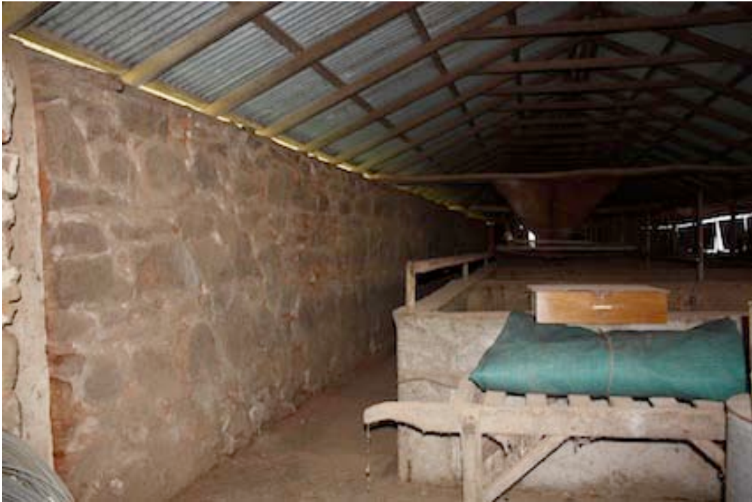
Figure 35 Interior view of Cart Shed, looking north. The concrete walls represent pig pens
