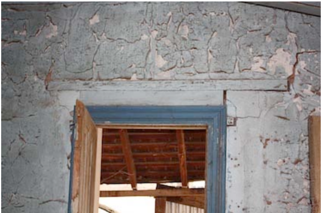
Figure 8 Detail of the door leading from the Bedroom to the Entertaining Room. Note the timber lintel above the door frame
