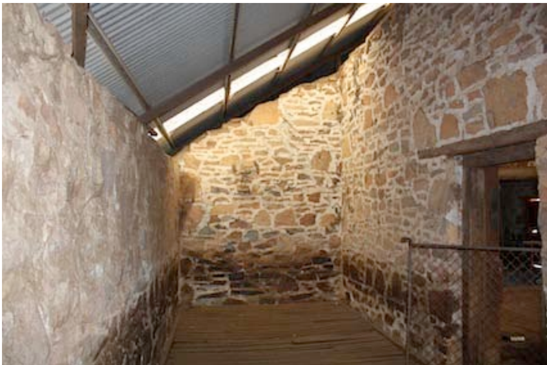
Figure 18 Interior of single storey section looking south. This is the room on the eastern side of the wool shed.
