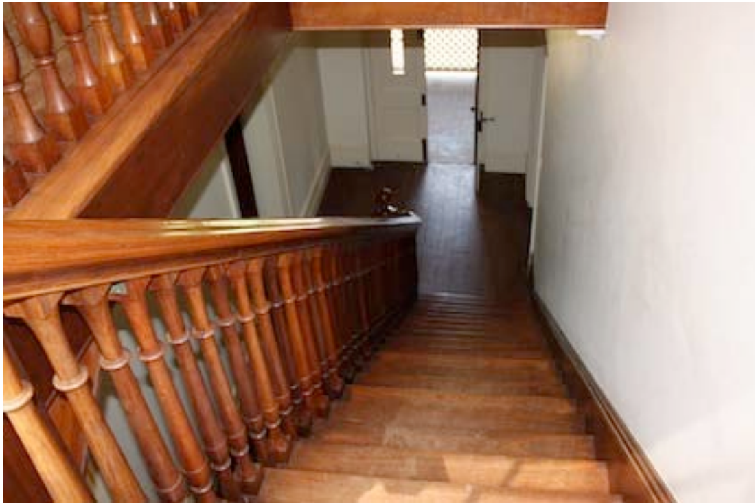
Figure 12 Staircase looking down to the ground floor and the main entrance on the southern side of the building.
