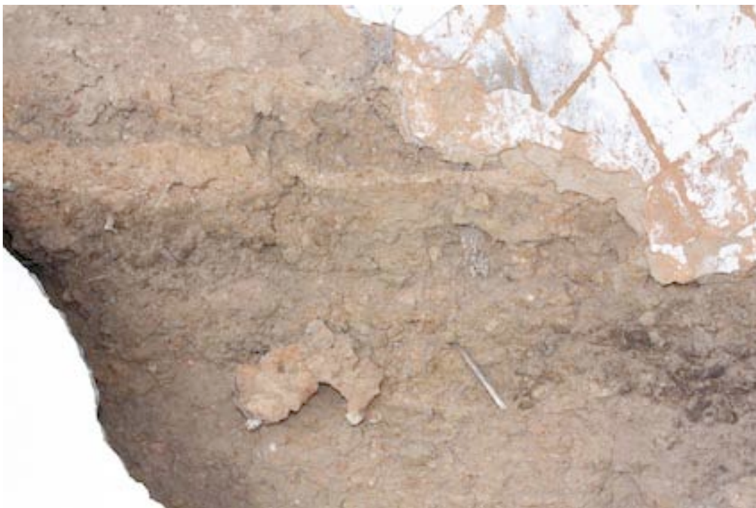
Figure 6 Detail of rammed earth wall where limewash render has become dislodged
