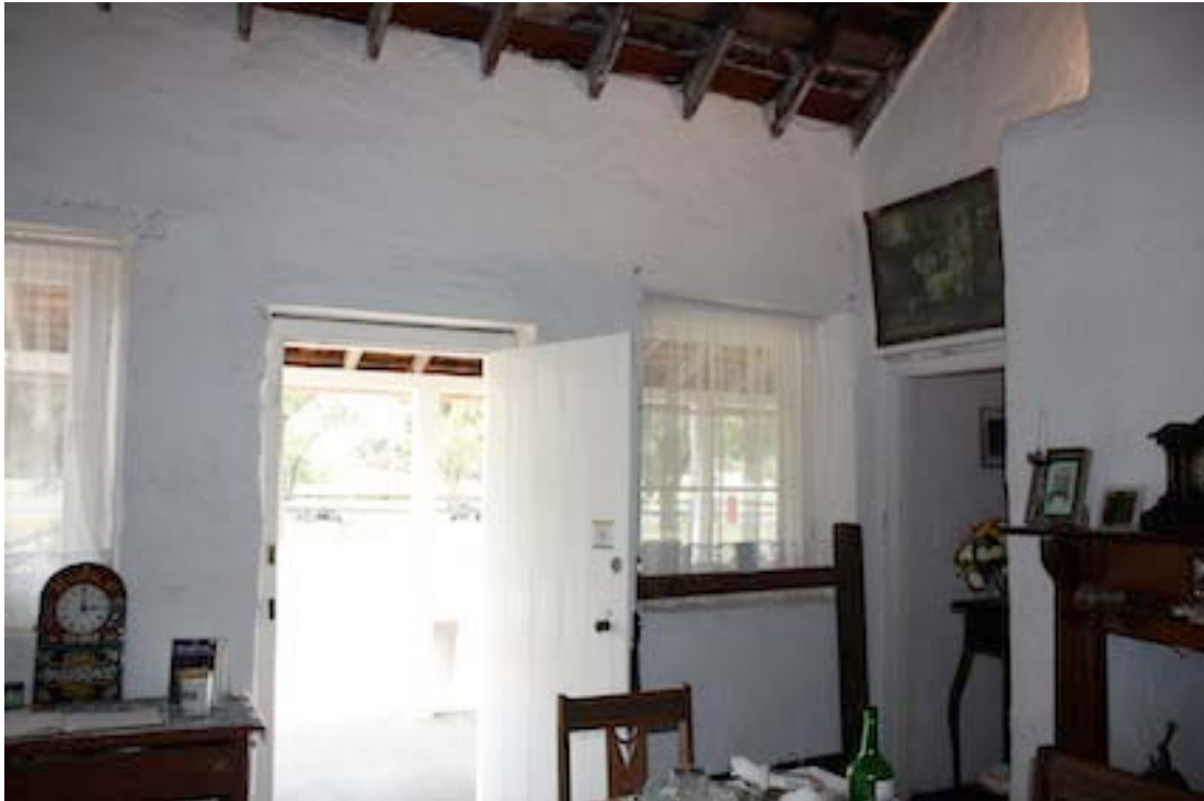
Figure 6 Interior of Room 1 looking towards front door. Door on the right leads to Room 2
