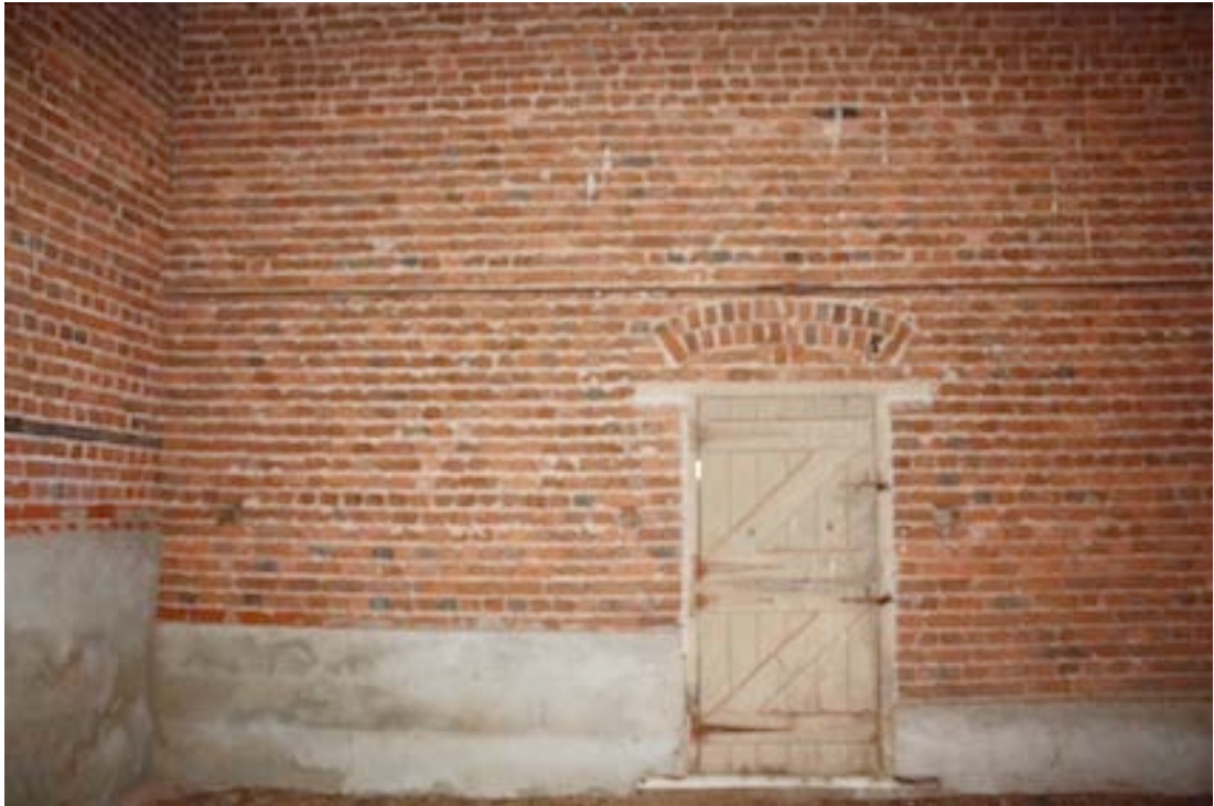
Figure 45 Interior of central room (shearing area) showing the less carefully laid bricks and the door leading into the room at the northern end of the building.
