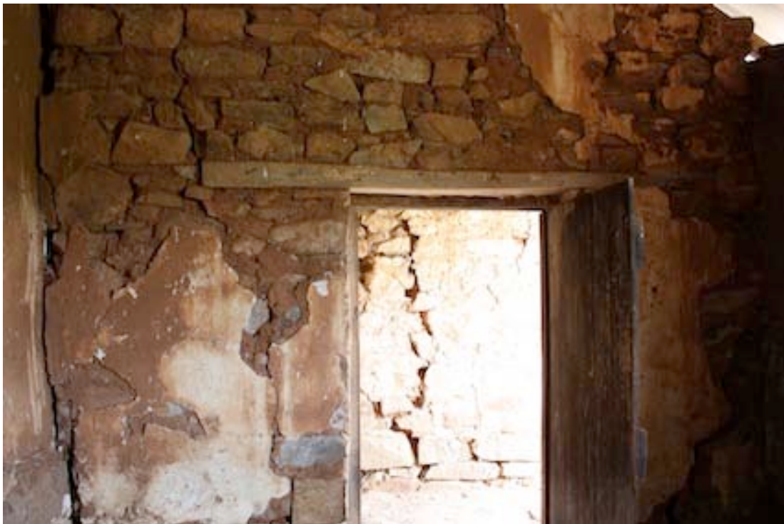
Figure 36 Doorway leading from the western saddle and harness room to the passage that leads between the northern and southern side of the building.
