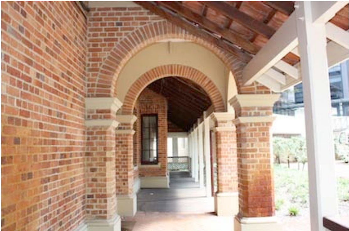
Figure 5 Northern elevation looking west towards arched portico and projecting bay containing secondary door.
