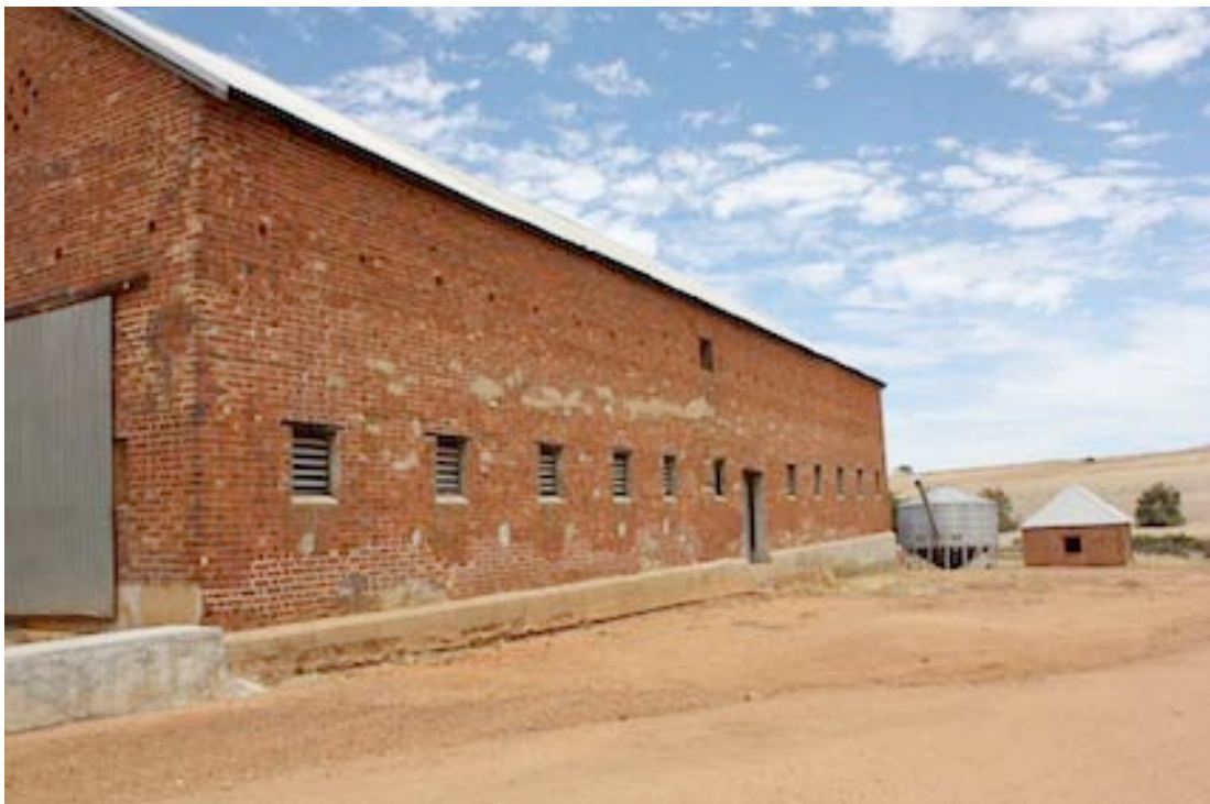
Figure 28 Northern side of the Stables. The windows along this side replace the earlier narrow windows. Note the lack of a brick arch to these windows compared to the narrow window on the southern side
