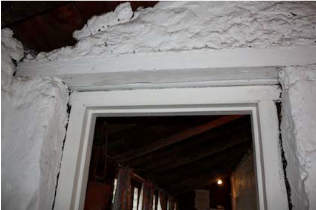
Figure 10 Detail of doorway leading from Room 5 onto the back verandah. Note timber lintel and the doorframe with mortise and tenon joint secured with timber peg
