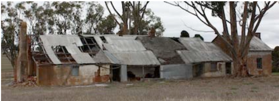
Figure 3 Western side of Homestead. The originally detached kitchen can clearly be seen on the right
