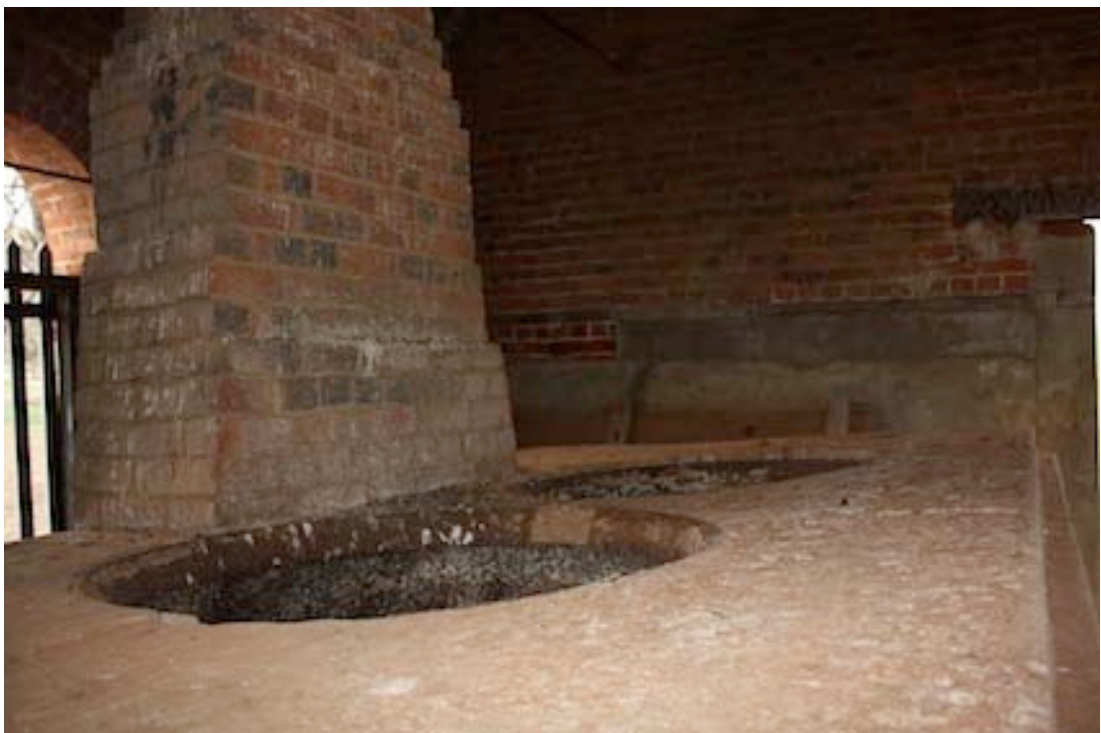
Figure 44 The coppers at the southern side of the building next to the sheep dip.
