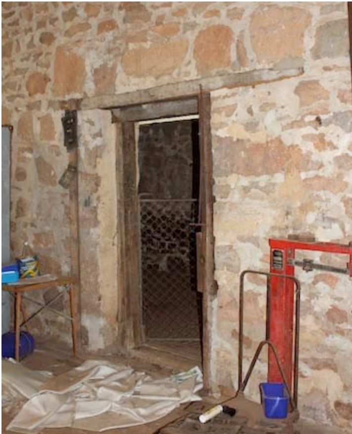
Figure 22 Door on the eastern side of the wool shed which leads into the narrow single storey room on its eastern side
