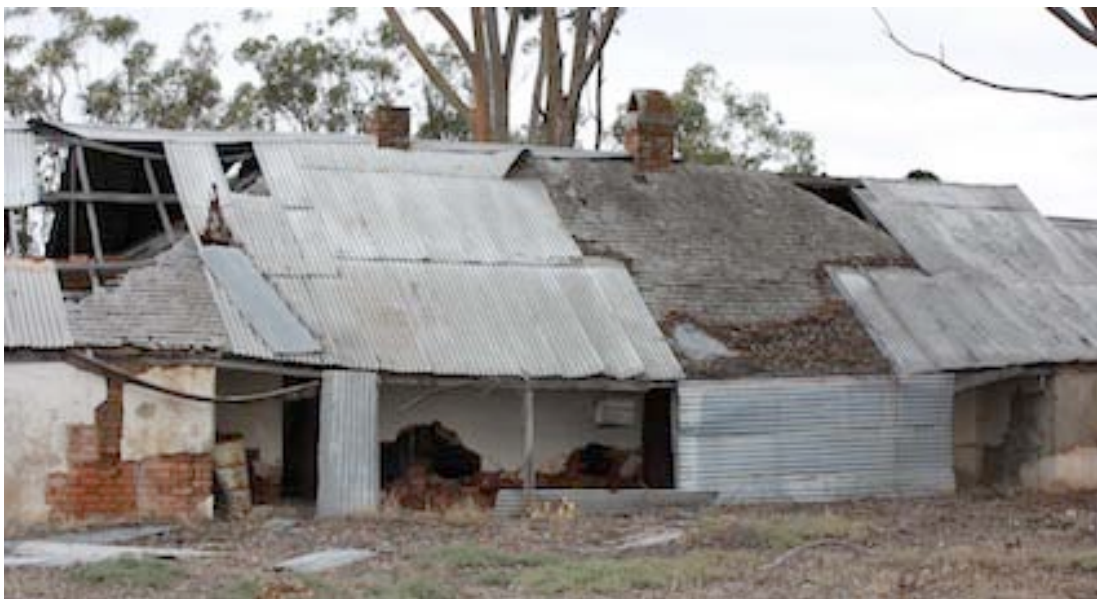
Figure 4 Detail of the original core of homestead which has retained the original hipped, shingled roof beneath later iron cladding
