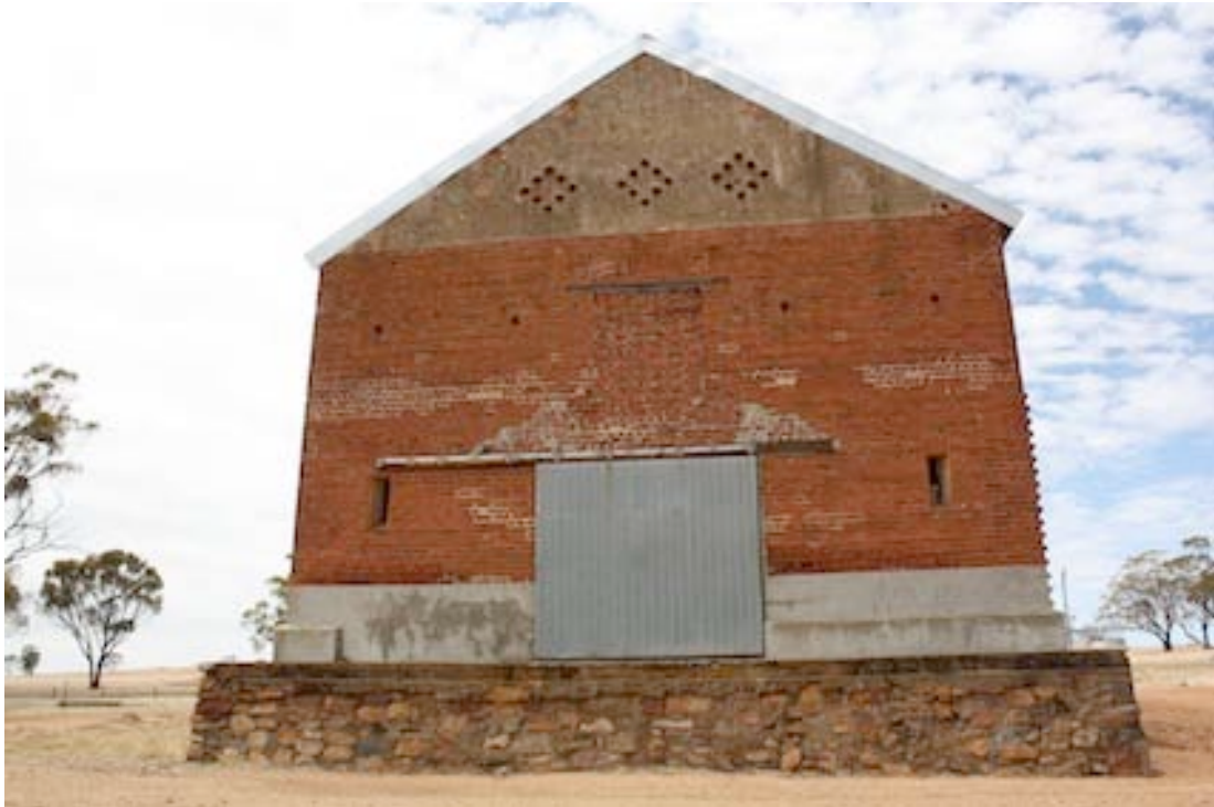
Figure 27 Western end of the Stables. The left doorway has been filled in but the round bricks have been retained. Note the irregular edge on the right hand side.
