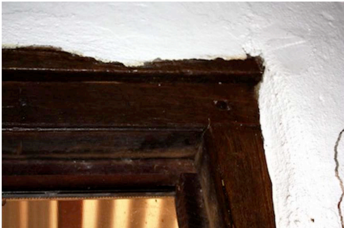
Figure 9 Detail of door joinery showing wooden dowel fixing mortise and tenon joint.
