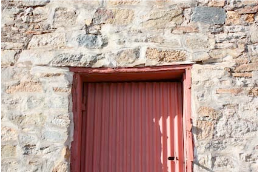
Figure 21 Door on the western side which leads into the mill area. Notice the sagging timber lintel
