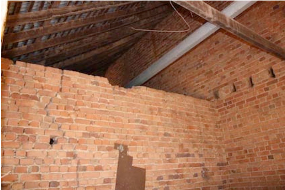
Figure 15 Interior of western single storey section, one of the rooms at the southern end. Note openings in the eastern wall that formerly held joists.
