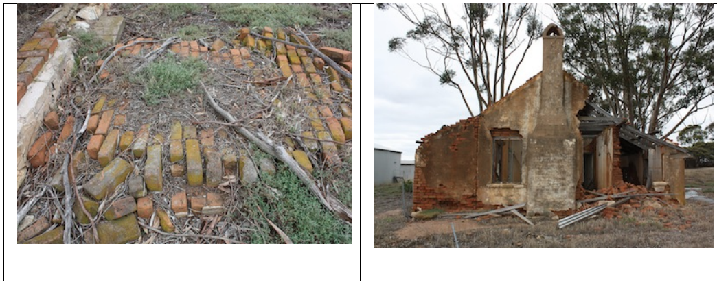
Figure 8.8 Buildings at 'Martinup'. Collapsed wall in the Men's Quarters on the left and the end wall on the Homestead on the right (F. Bush 10 February 2011)
