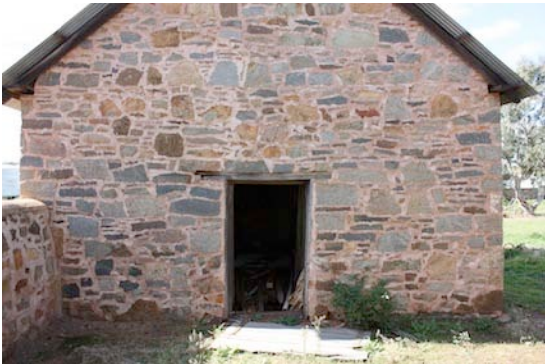
Figure 11 Western wall. The timber lintel supports the stone work for the doorway
