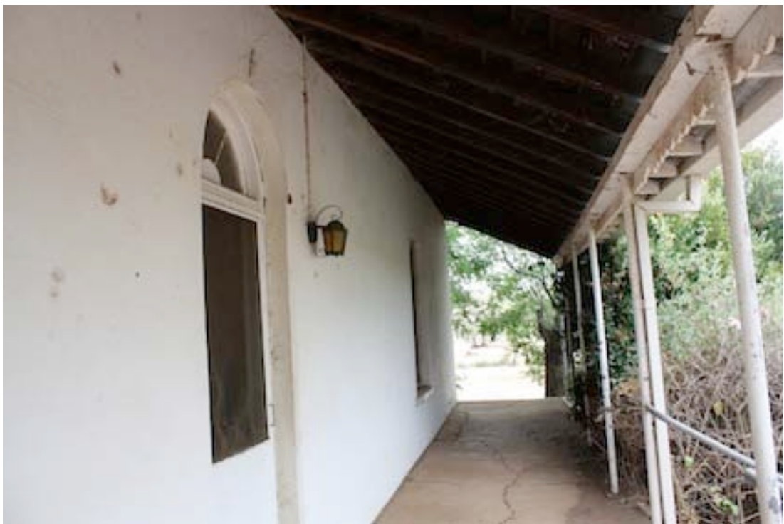
Figure 5 View of front verandah looking west. Note round arched fanlight to main door
