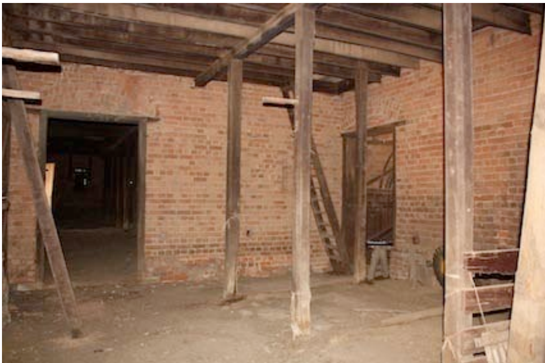
Figure 16 Interior view of two storey section looking south. On the right is the entrance from the western side of the building and the ladder to the loft. The door leads to the southern half of the building.
