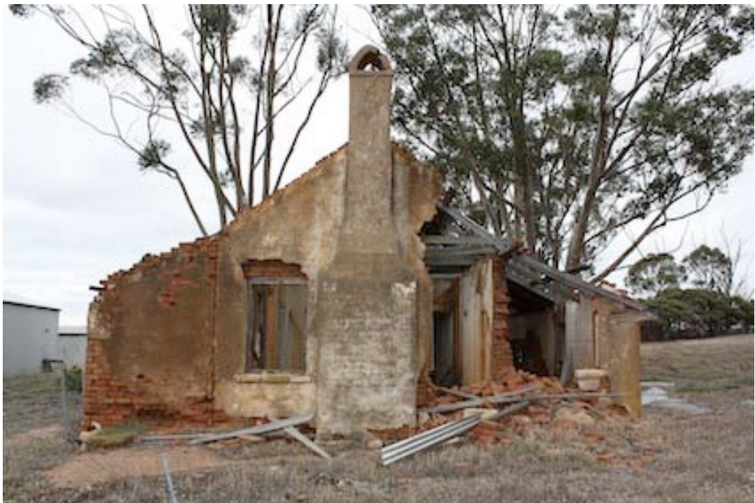
Figure 6 Northern end of Homestead showing the collapsed wall of the Entertaining Room
