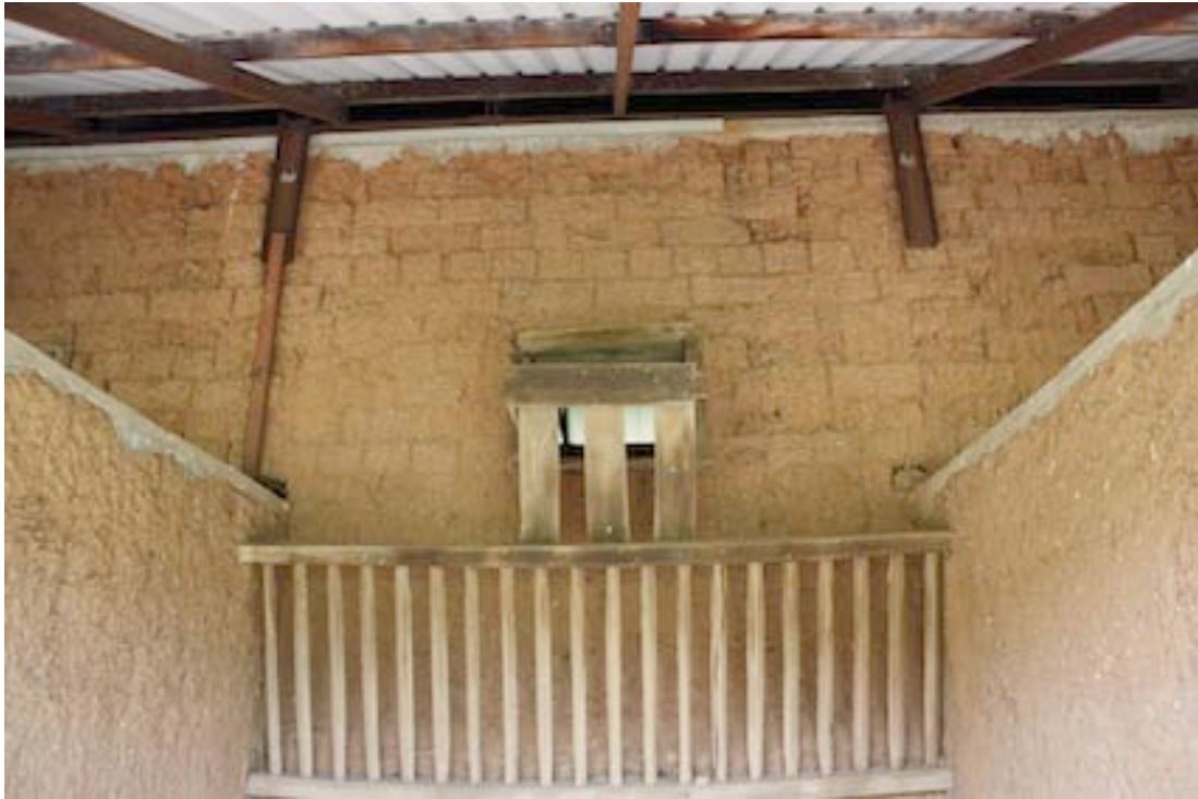
Figure 35 Horse stalls on the northern side of the building. Note the cob dividing walls.
