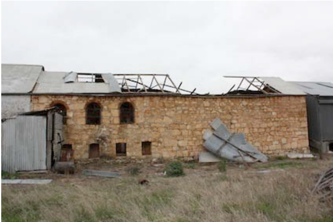
Figure 26 Western side of Shearing Shed with new steel shed on the right
