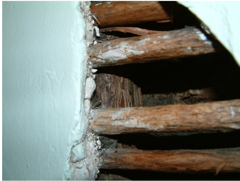
Figure 4.2 Section of wattle and daub walling, Patrick Taylor Cottage, Albany (F. Bush 3 July 2008)
