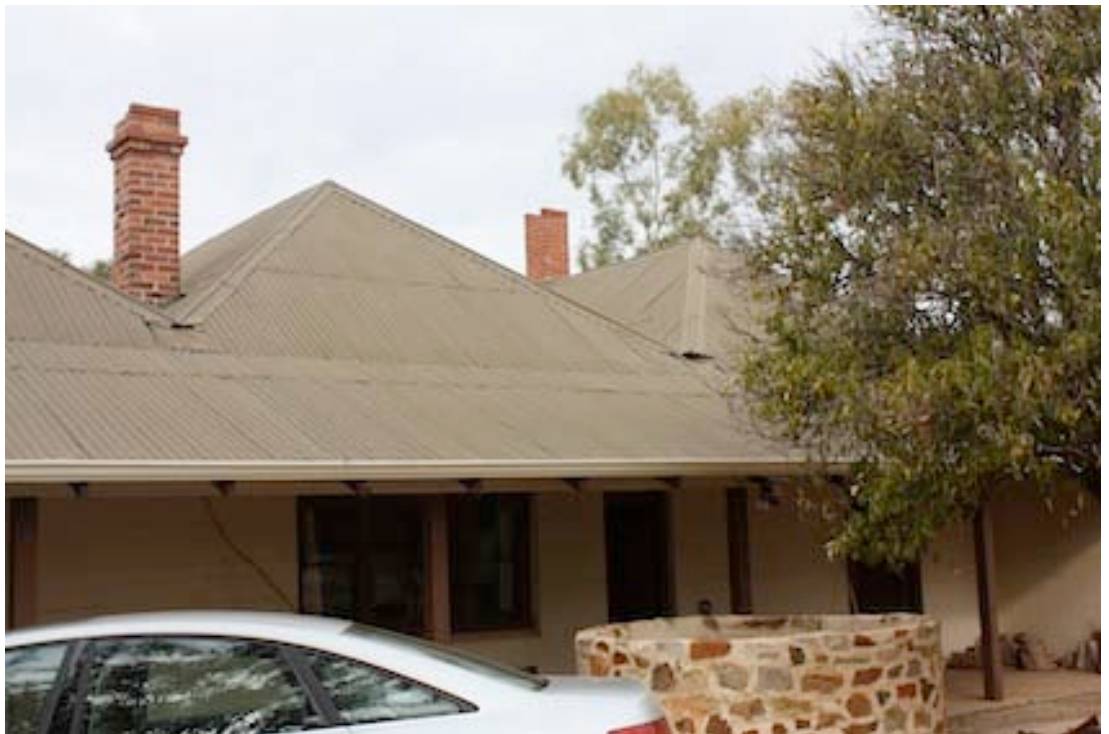
Figure 3 Detail of front showing the three hipped roof sections and chimney stacks
