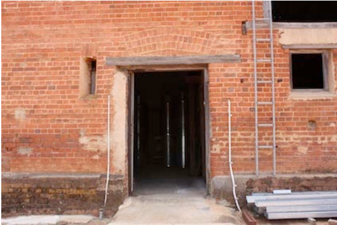
Figure 29 Detail of southern side of window showing brick arch to doorway and also to the narrow window.
