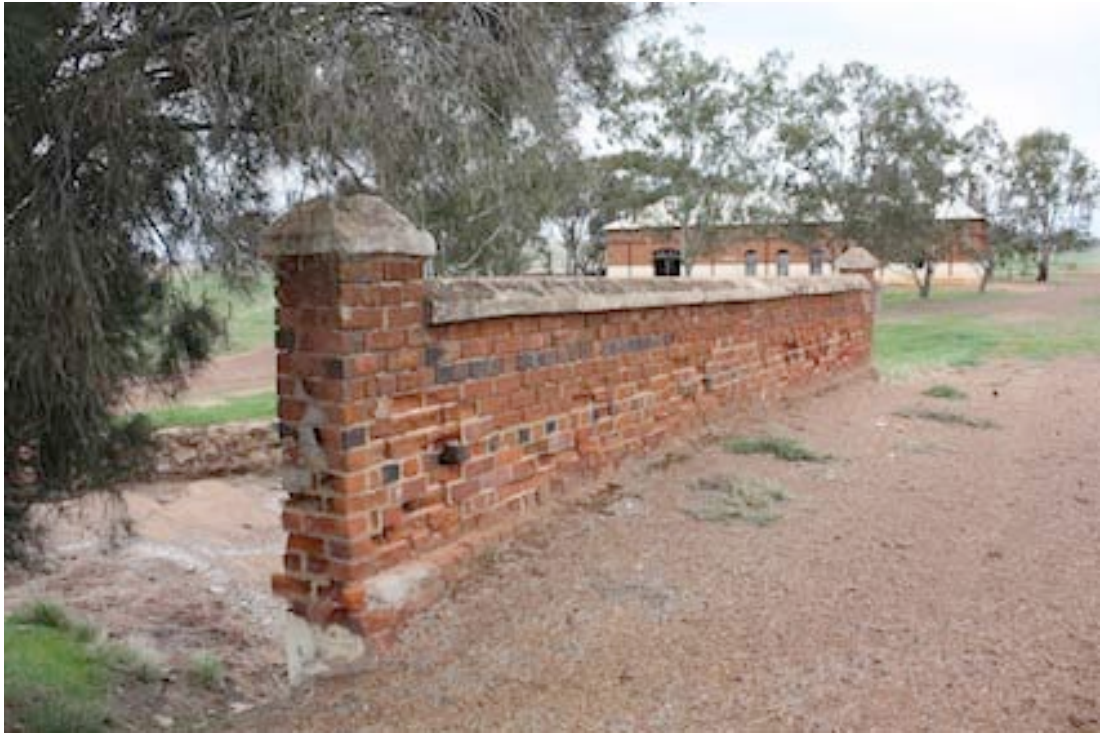
Figure 49 Southern side of bridge looking west towards the Shearing Shed and the main road.
