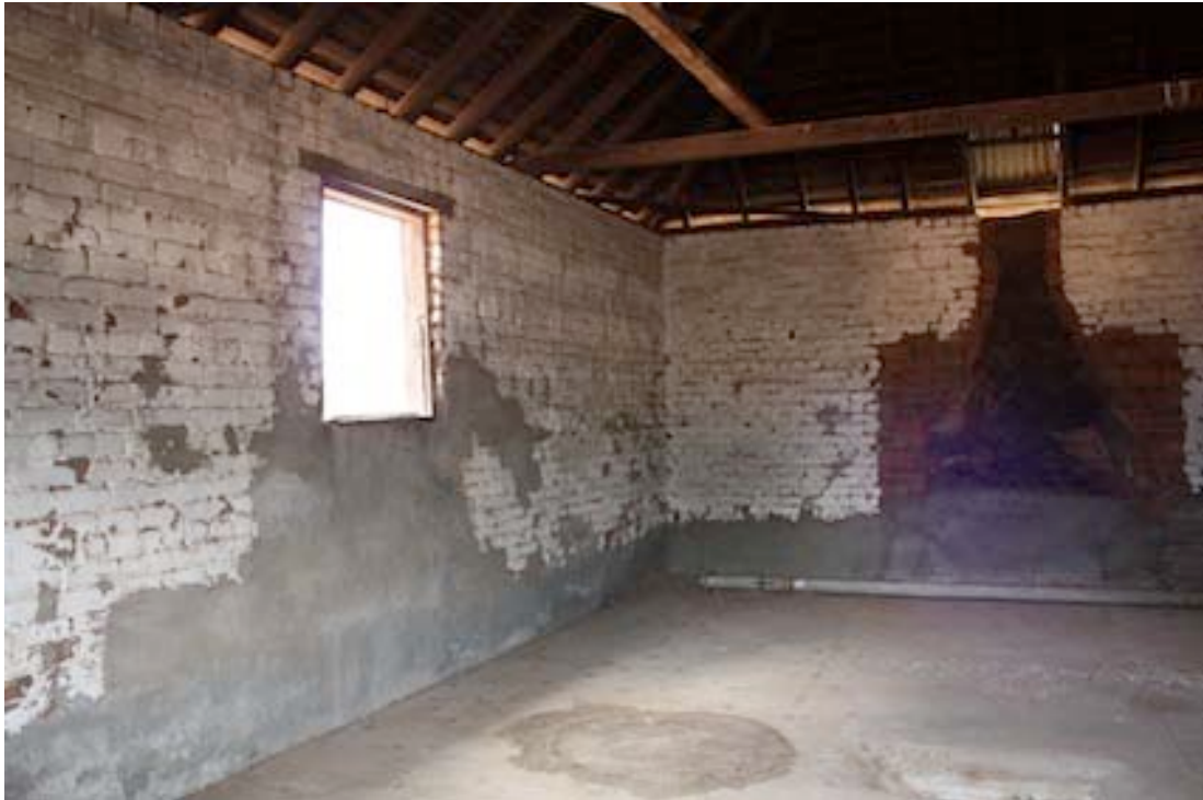
Figure 22 Interior view of Workers' Quarters looking south. The previous location of the chimney and fireplace can be seen in the west wall at the rear.
