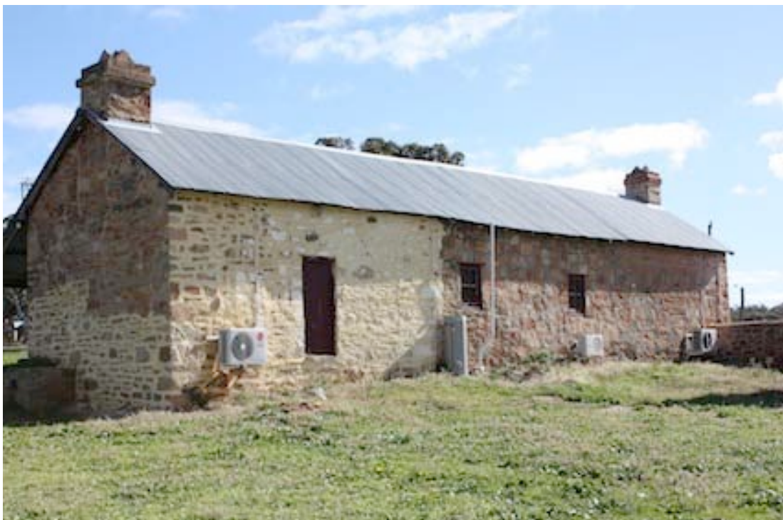
Figure 4 Eastern side of the Kitchen Stores looking north towards the east-west wall that butts up against the eastern wall of the Kitchen Stores at the eastern wall of the Bulk Store
