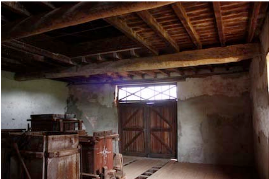
Figure 46 Room at the northern end of the building. Note the bush pole girders and the flooring members above.
