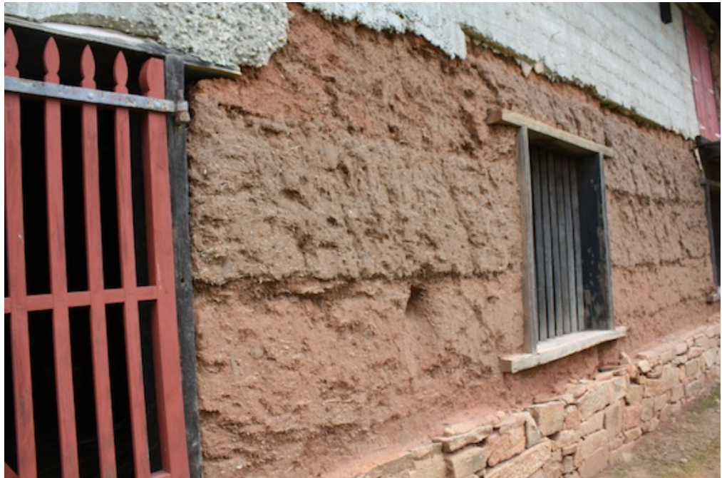
Figure 4.3 Stables at 'Berkshire Valley' the lower section of the wall is an example of cob walling due to the inclusion of straw in the mix (F. Bush 11 August 2010)
