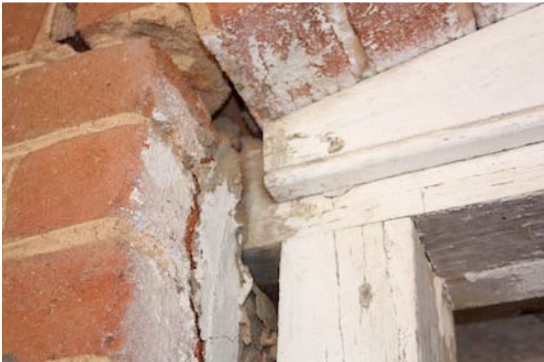
Figure 16 Detail of door frame on northern side of building which shows the mortise and tenon joint
