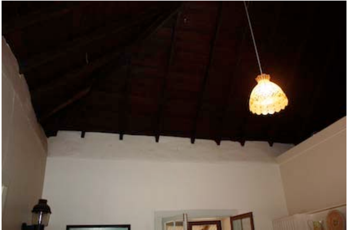
Figure 16 Detail of eastern wall in Room 4 showing extension to the wall and the rafters. The doors lead out to the rear verandah
