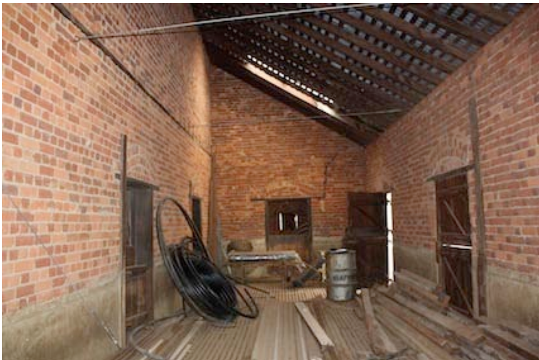
Figure 25 Interior view of western section of shearing shed looking south. Note slatted timber floor.
