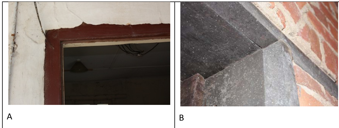
Figure 8.18 The image on the left shows a mortise and tenon joint secured with a wooden dowel (Gwambygine c.1836). The image on the right (Shearing Shed at ‘Glentromie’ 1870s) shows a butt joint (F. Bush)
