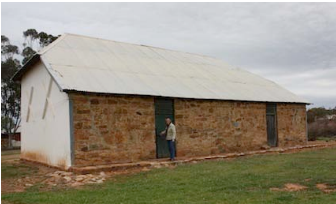
Figure 6 Rear view of Mill Building looking towards the north-east corner of the building. Note wall ties.
