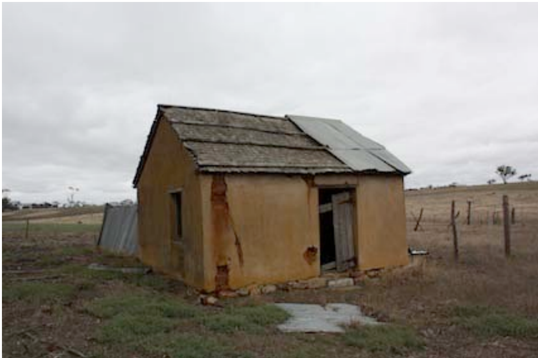
Figure 18 South-east corner. Note the stone foundation and the original shingle roofing material that survived beneath later iron cladding
