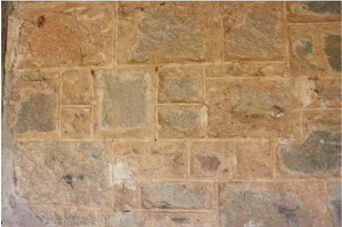
Figure 5 Detail of stonework on the western side of the Kitchen Stores. This stonework has been marked out to resemble dressed stonework.
