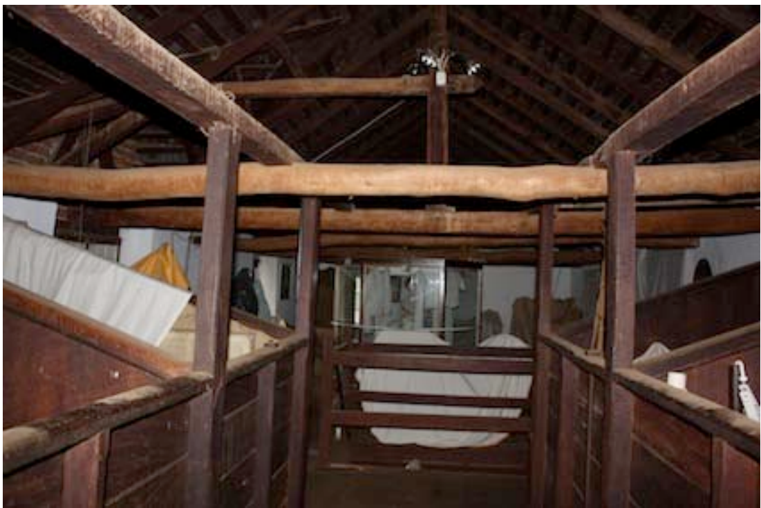
Figure 8 Interior view of upper floor looking east towards bins. Note bush pole ties.
