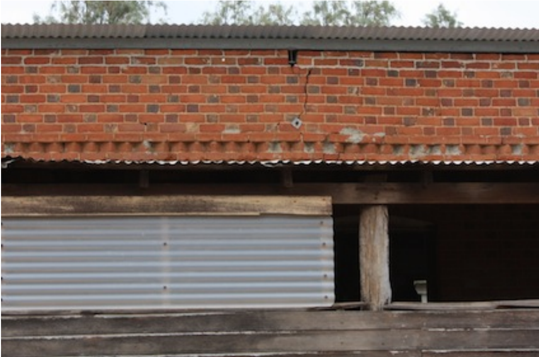
Figure 8.13 Detail of saw-tooth pattern above the line of the verandah roof of the Shearing Shed (F. Bush 19 December 2010)
