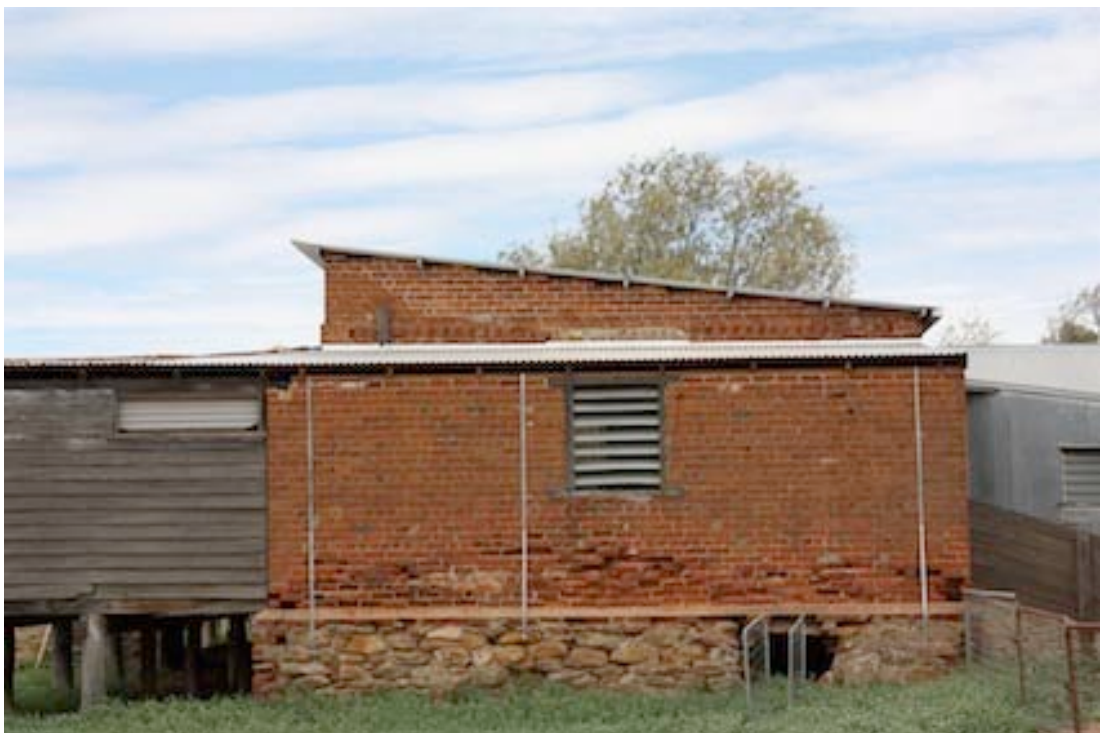
Figure 12 View of western end of Shearing Shed. A single row of saw-toothed edged bricks can be seen just above the line of the roof of the side addition
