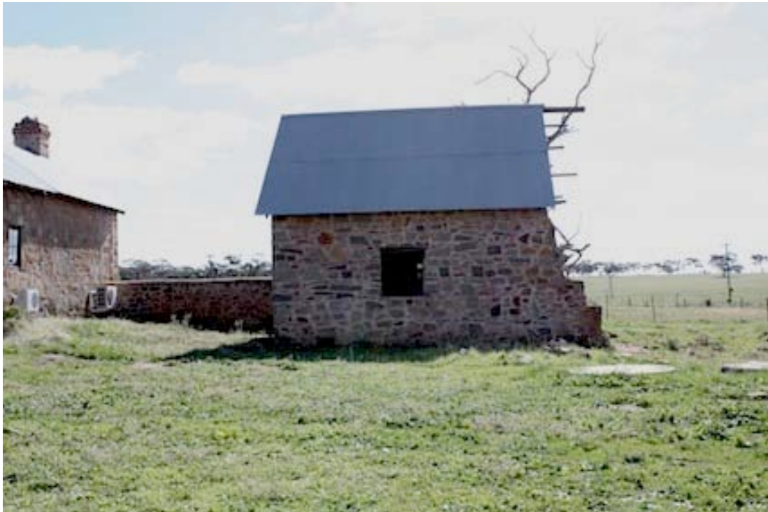
Figure 10 Southern side of building. The exposed rafters and jagged wall on the right, indicates the former location of the quarters. Note the wall that runs between this building and the Kitchen Stores.
