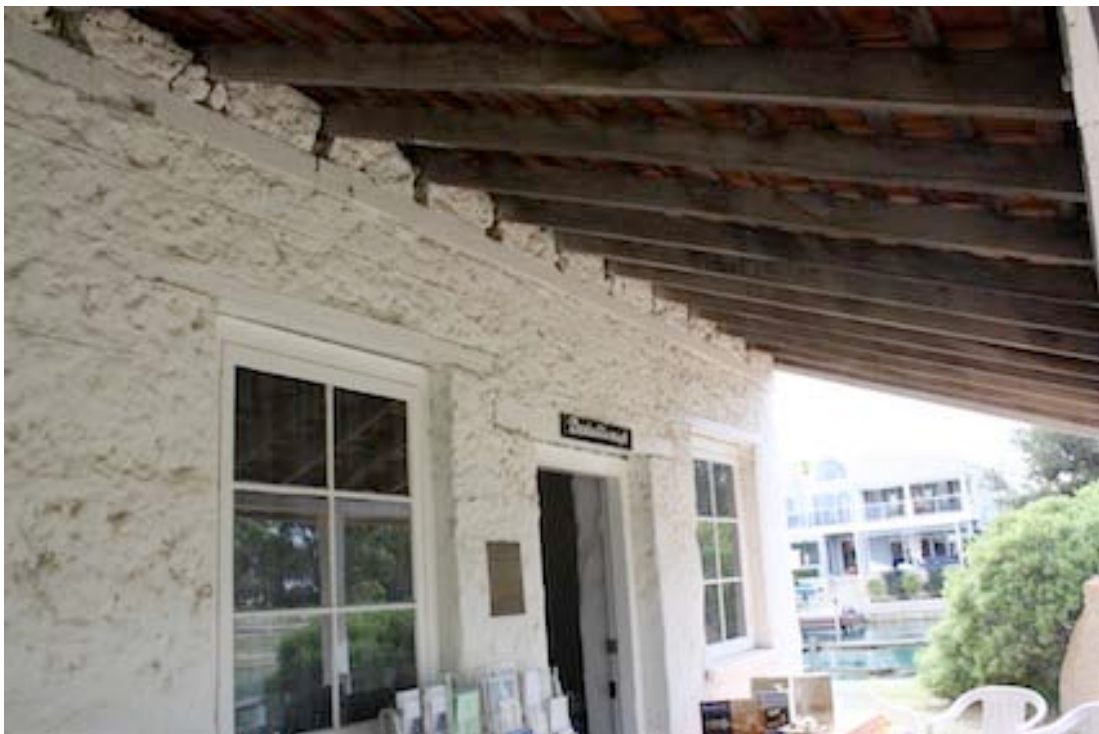
Figure 5 View of front verandah. Note additional layer of stonework above timber plate at top of the wall and timber lintels.
