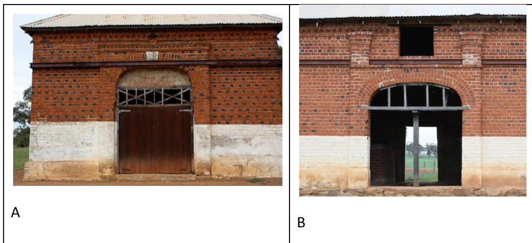
Figure 8.14 Shearing Shed at 'Berkshire Valley', A is northern end, B is the entry in the east wall (F. Bush 11 August 2010)
