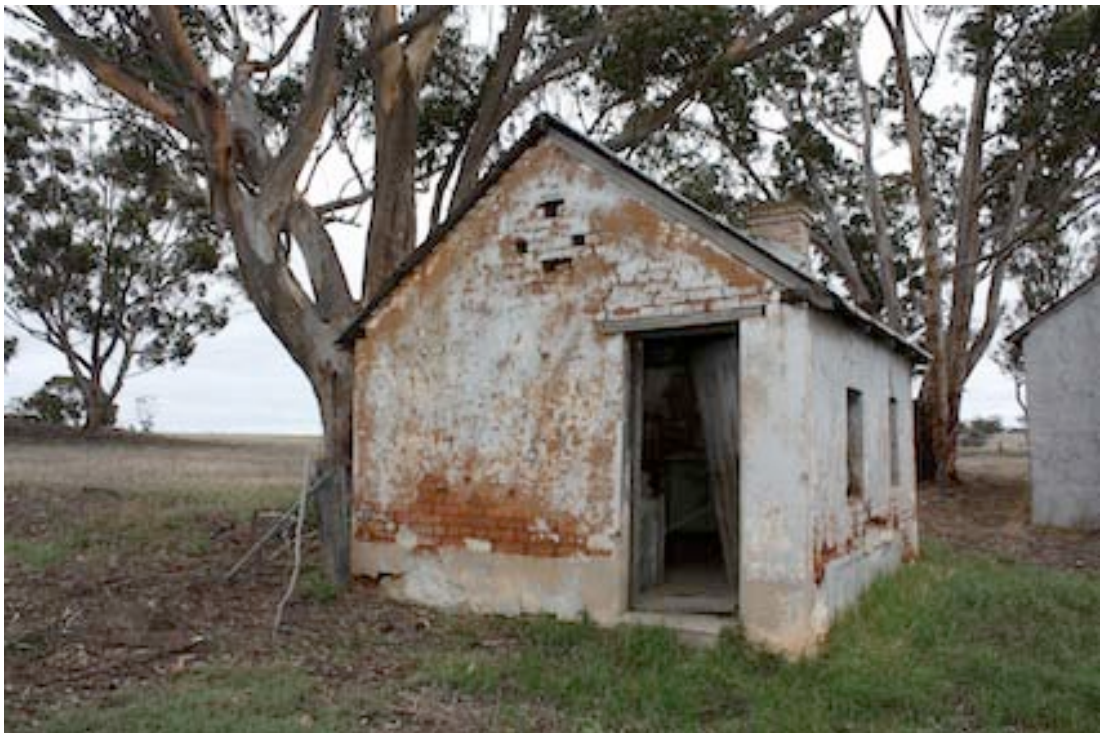
Figure 12 Southern end. Note ventilation in gable end and the timber lintel that spans the door opening.
