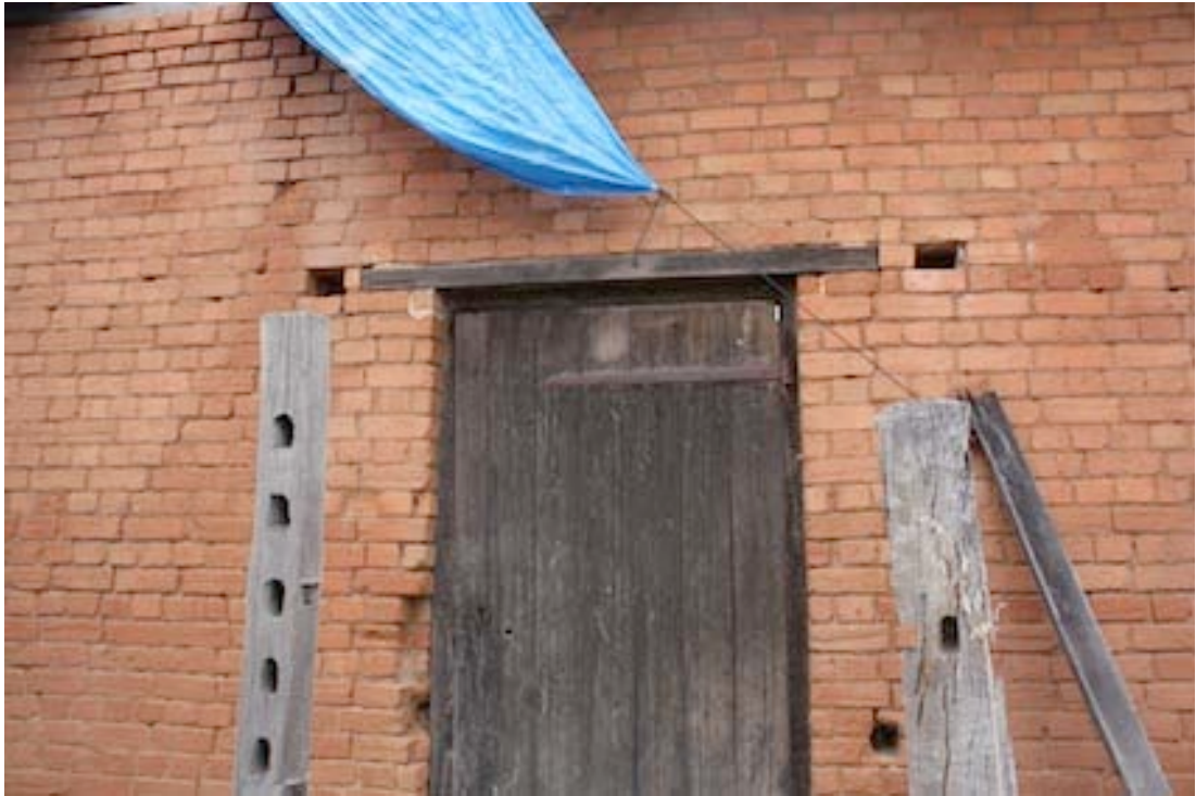
Figure 24 Detail of door on northern side of Wool Barn. Note lack of relieving arch
