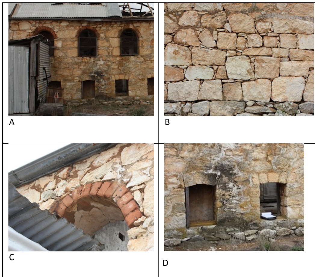
Figure 8.6 'Martinup' Shearing Shed (A), detail of stonework (B), arch to upper opening (C), lower opening (D). (F. Bush 10 February 2011)
