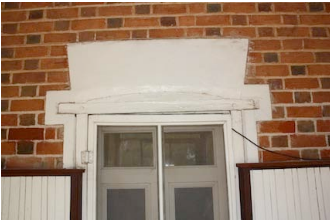
Figure 16 Detail of French doors at the western end of the building. Note timber dado covering bricks and the door frame with mortise and tenon join secured with a dowel.
