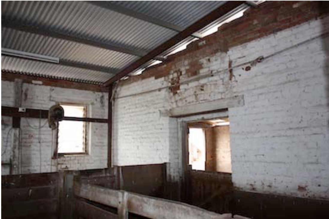
Figure 15 Interior view of the Shearing Shed looking north towards the side addition. Note brick arch above the timber lintel
