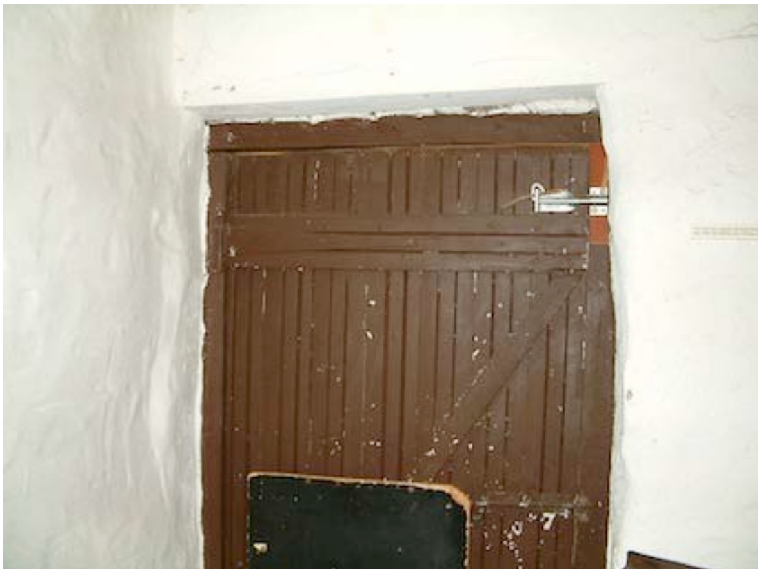
Figure 11 Doorway on the western side of Room 3 leading to the exterior. The door is not original
