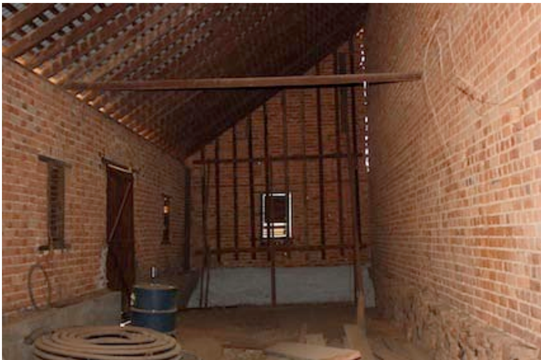
Figure 14 Interior of western side looking north; note bracing to north wall. On the right is the western wall of the two storey section.
