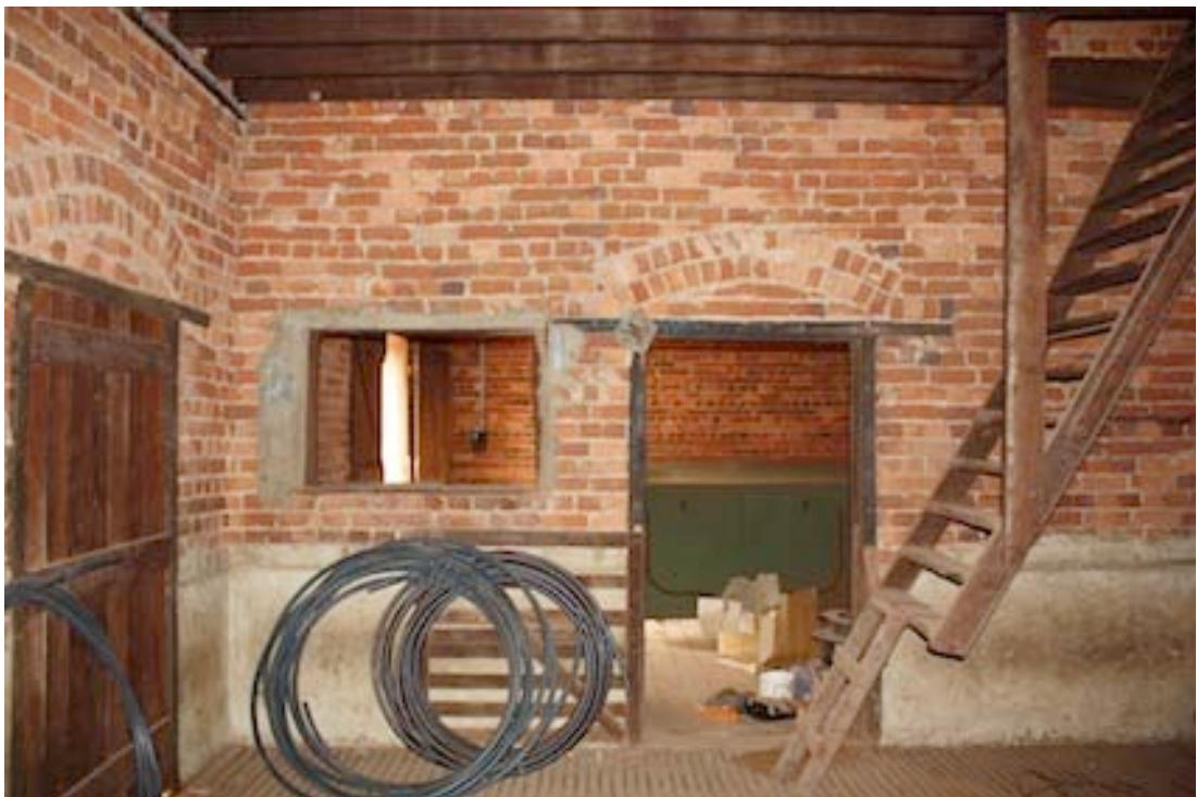
Figure 27 Eastern side of shearing shed looking south towards ladder to loft area and rooms at the southern end of the building.
