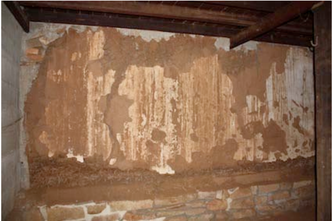
Figure 33 Interior view showing one of the interior cob walls in the southern section.
