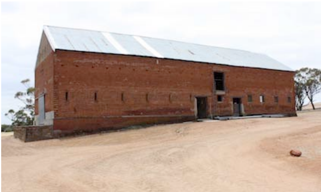
Figure 26 Southern side of Stables showing row of round bricks to the first floor and the original narrow windows on the ground floor at the western end of the building.
