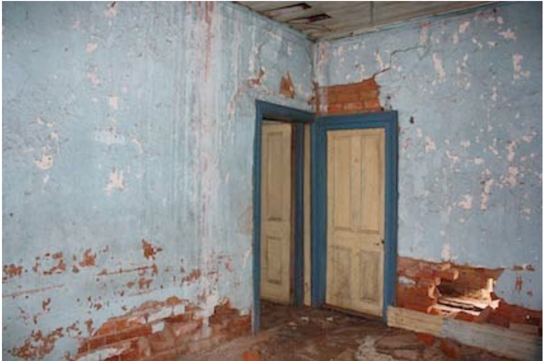
Figure 7 Bedroom looking towards the south-west corner with doors leading to the exterior and the Sitting Room
