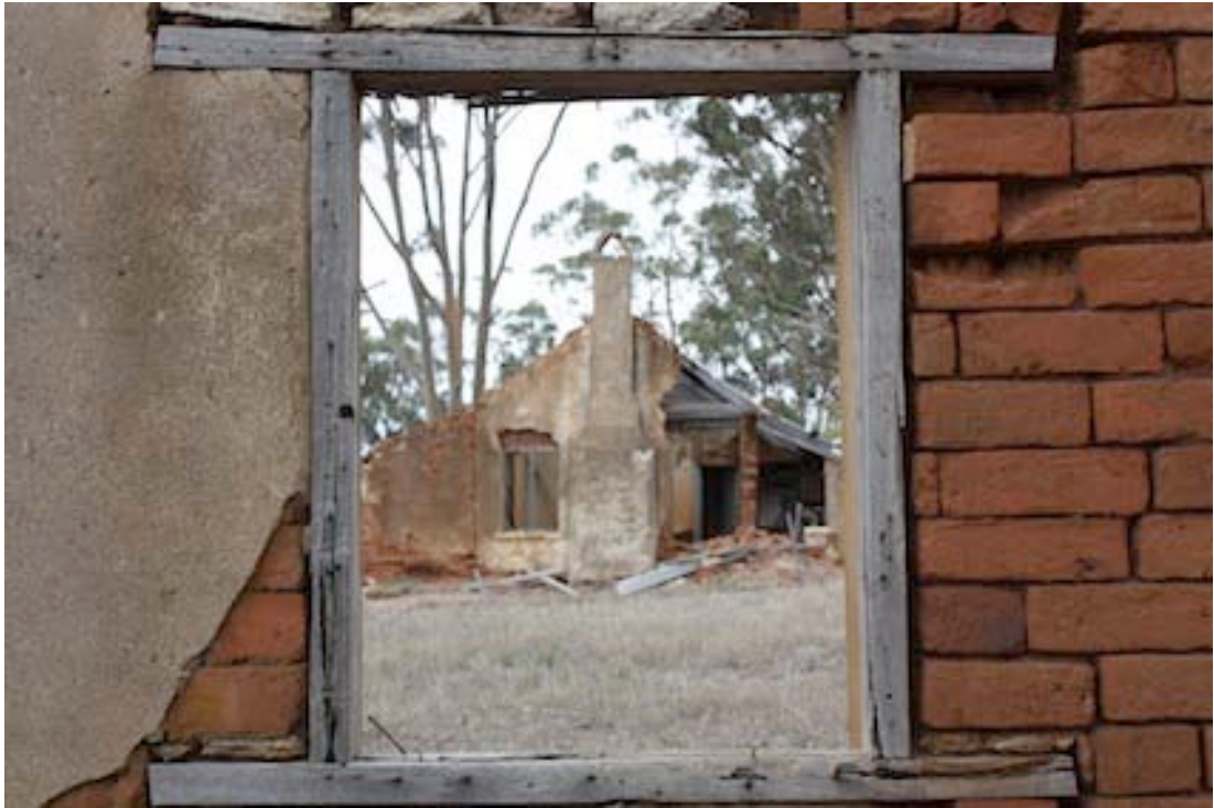
Figure 16 Window in eastern wall, looking towards the Homestead. Note butt joints to window frame
