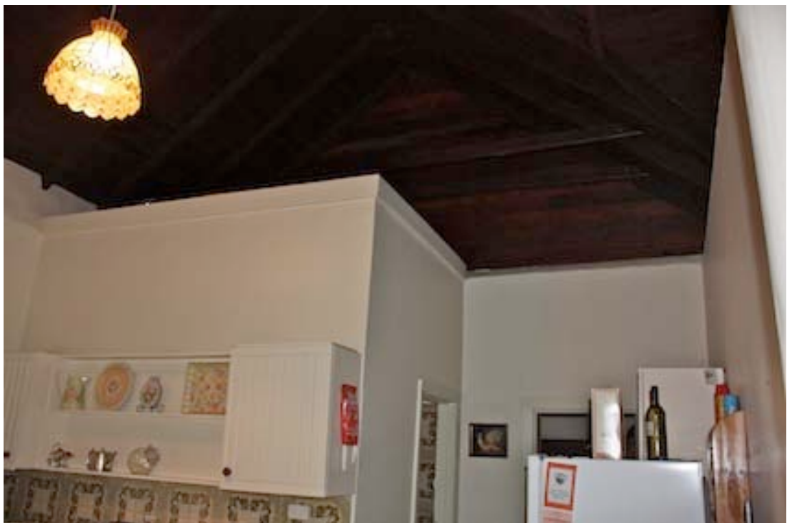
Figure 15 Interior view of Room 4 (kitchen) looking south towards the bathroom that has been built in this large room
