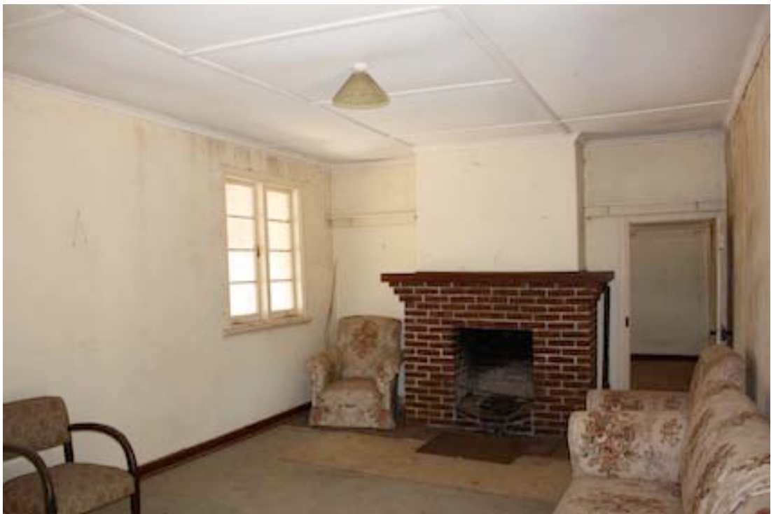
Figure 9 Room 13 looking south towards doorway to Room 14. Note new fireplace surround and casement window
