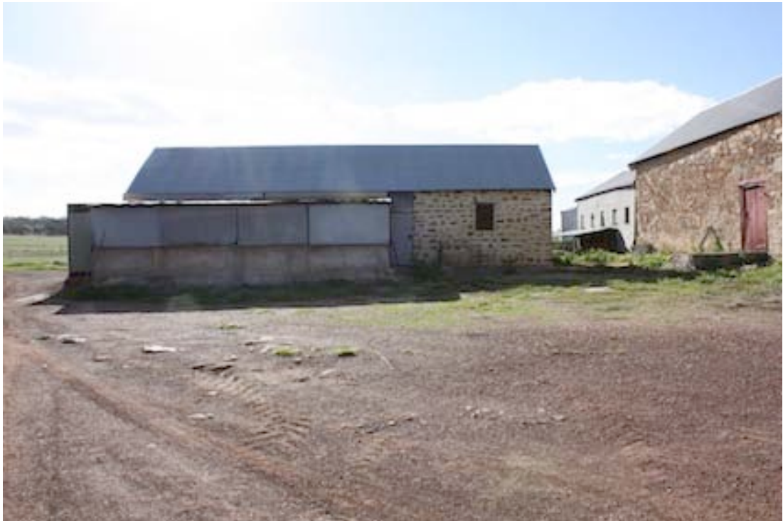
Figure 24 Southern side of Stables with the more recent concrete and galvanised iron section on the left side of the building
