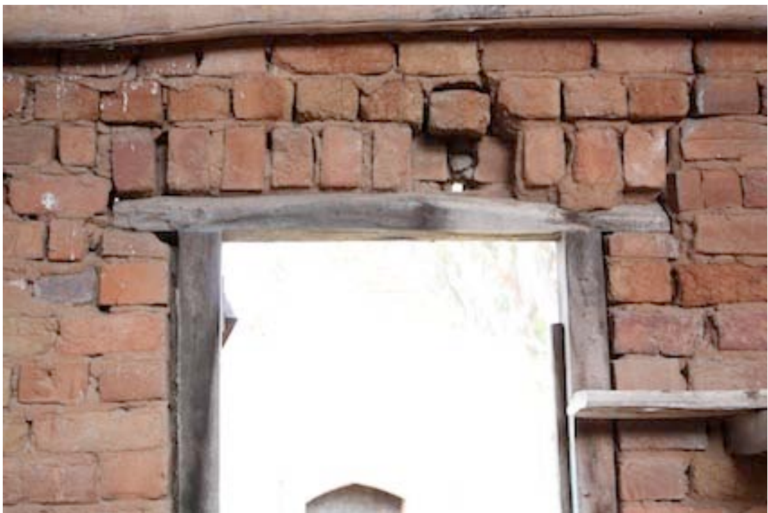
Figure 20 Detail of window in southern wall. Note the use of header bricks to create a relieving arch over the window's timber frame and the use of butt joints.
