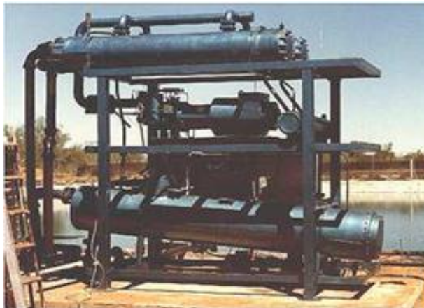
Figure 2.8 ORC engine installed in Alice Spring solar pond
