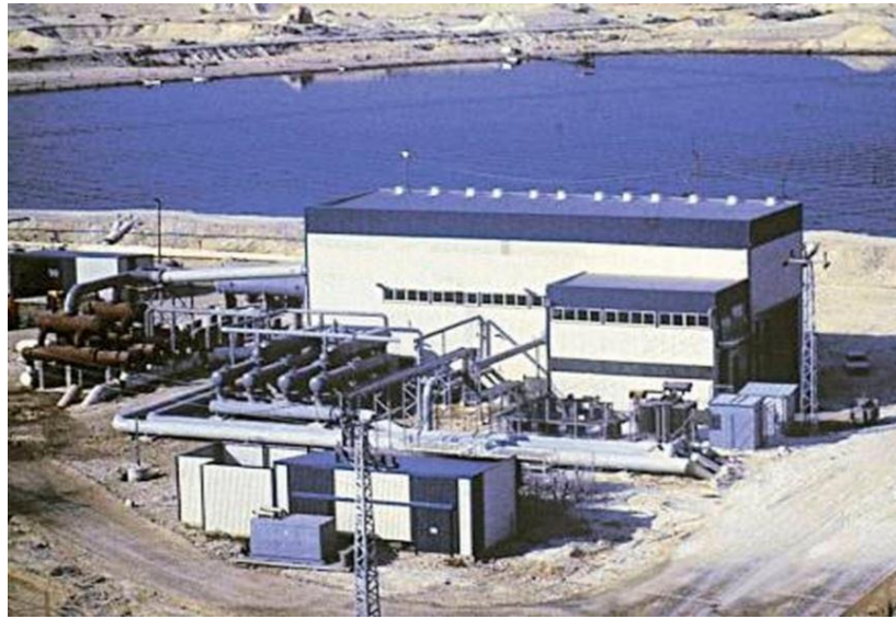
Figure 2.12 The Beith Ha'rava solar pond power plant (SPPP)
