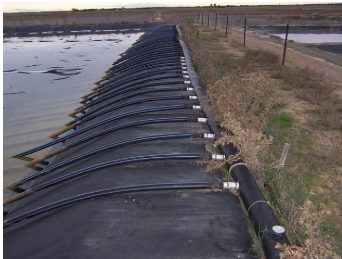
Figure 2.5 In-pond heat exchanger at Pyramid Hill solar pond
