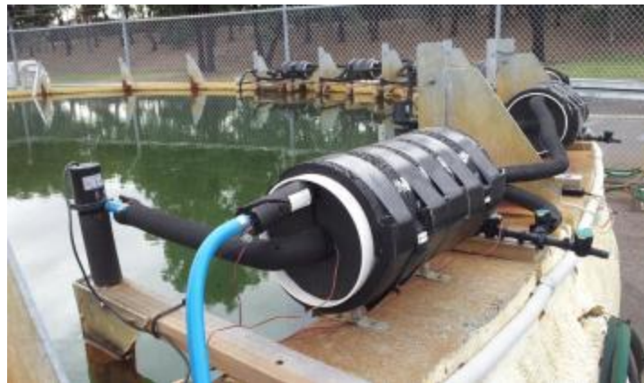
Figure 4.16 Insulated heat exchangers (HEX)
