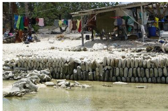
Figure 15: Private residence sea wall, 2011
