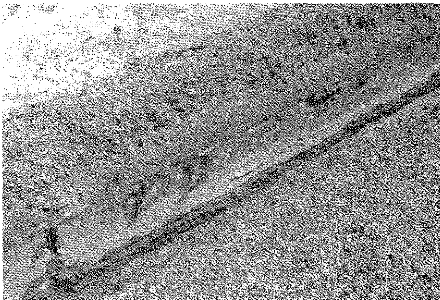
Joint # 13. Pavement edge exposed during subdrain removal. The light area on the edge of the pavement is grout.
