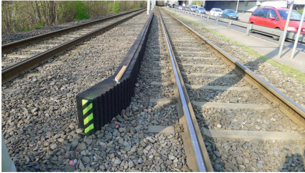
FIGURE 8. MNAS seen from the start of the section – chamfered first unit is evident in the front.
