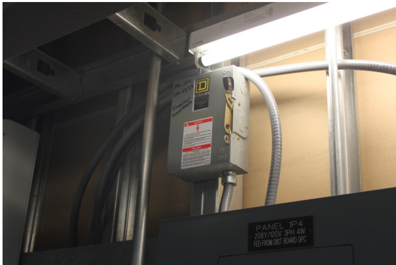
Figure 7: AC Disconnect in Equipment Room
