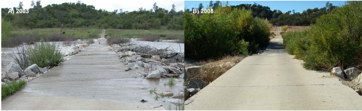
Figure 3.10: Concrete crossing on the Multi-Purpose Range Complex, Fort Hunter Liggett in A) 2003 with minimal vegetation growth and in B) 2008 with excessive vegetation growth.
