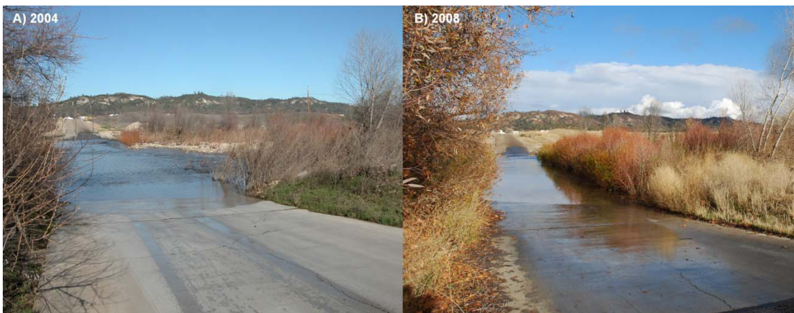
Figure 3.9: Concrete crossing on Del Venturi Road, Fort Hunter Liggett in A) 2004 following removal of stream vegetation, and in B) 2008 with stream channel occluded by vegetation.
