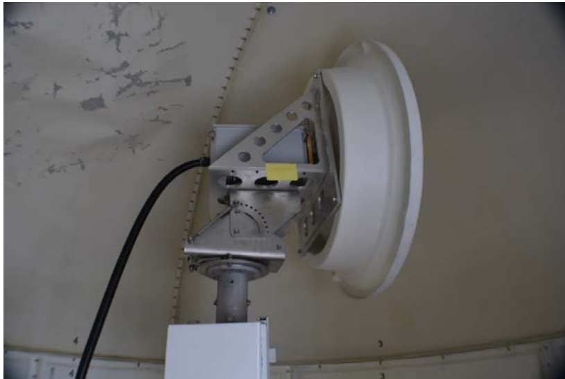
Figure 2. Photograph of 1.2-m antenna mounted inside radome at SG61.
