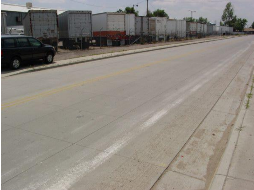
Figure 2.10 Typical Pavement Conditions Observed at Santa Fe Drive Site (Sheehan et al. 2004)
