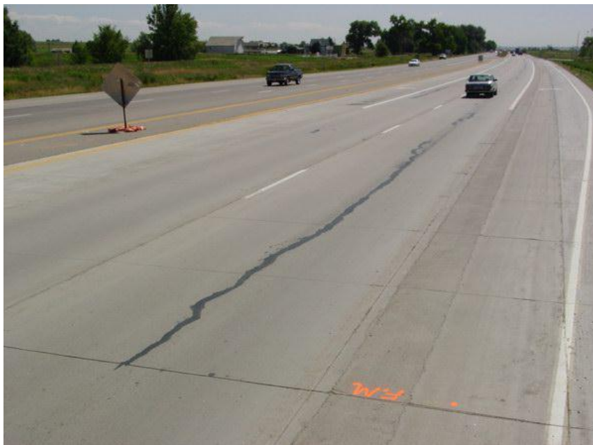
Figure 2.13 Typical Slab Cracking Observed in S.H. 119 Test Section No. 2 (Sheehan et al. 2004)
