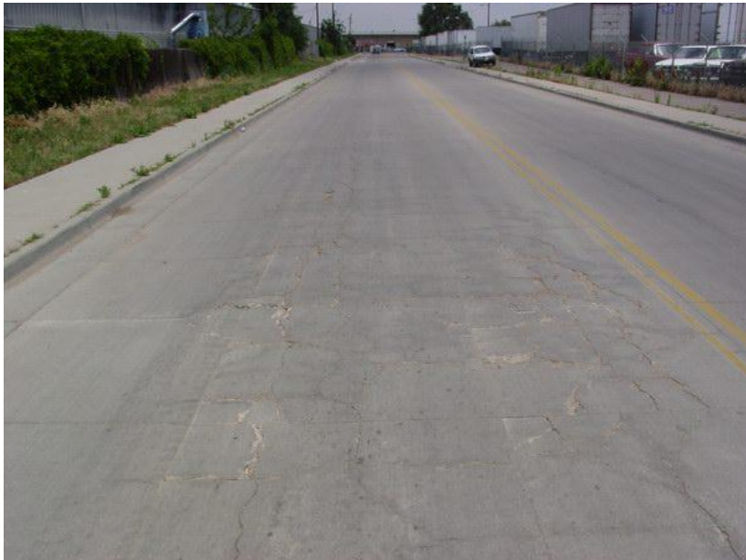
Figure 2.11 Stop Sign Approach Distressed Area Observed at Santa Fe Drive Site (Sheehan et al. 2004)
