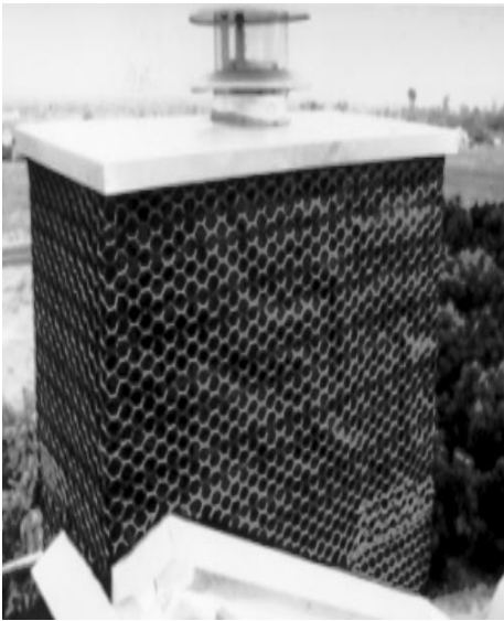
Fig. 23. Chimney with metal stack, heavy screen (animal excluder and spark arrestor), and tight roof to wall and Z-bar flashing joints.
