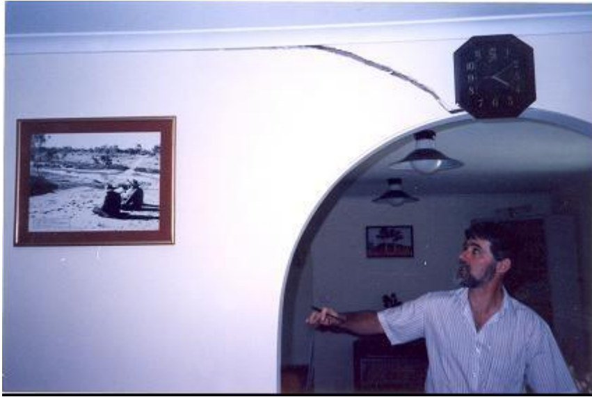
Figure 3 Crack on the Interior Wall between Dining Room and Lounge
