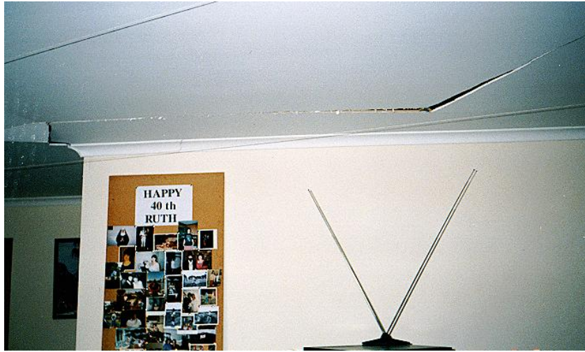
Figure 2 Crack on Ceiling in Family Area
