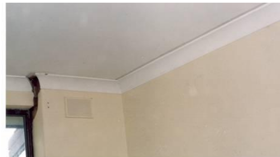
Figure 5 Distortion of Cornice in Laundry Area
