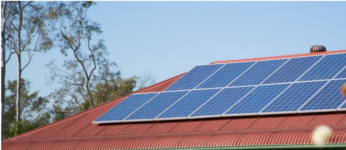
Figure 1.12: Solar PV on a residential house rooftop in Australia
