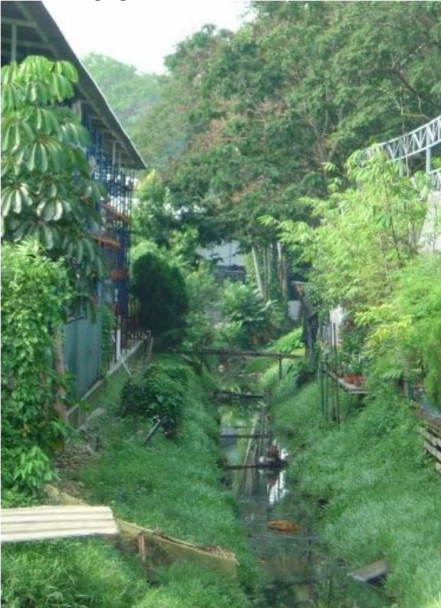
Fig. 15: Outlet Drain Condition @ Joan Rd [S'pore]
