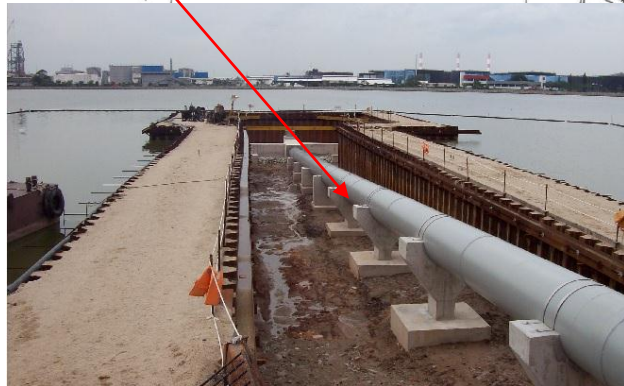
Fig. 20: Pumping Station & Discharge Point (Singapore)
