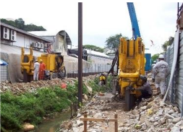
Fig. 16: Sheet Pile Installation Work to Widen & Deepen For the Improvement of existing Outlet Drain
