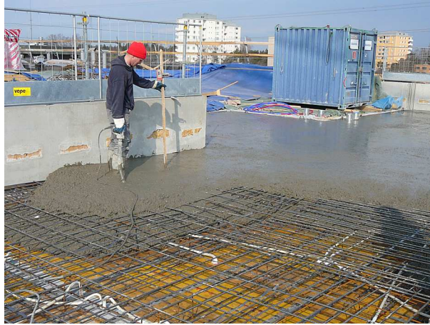
Figure 2.5: Placement and compaction of concrete around embedded steel reinforcement on a rooftop in Helsinki, Finland.
