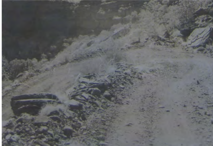
Figure 27: Section of the road to the mine. N.A.A Perth: Dept of Civil Aviation File 67/1265.
