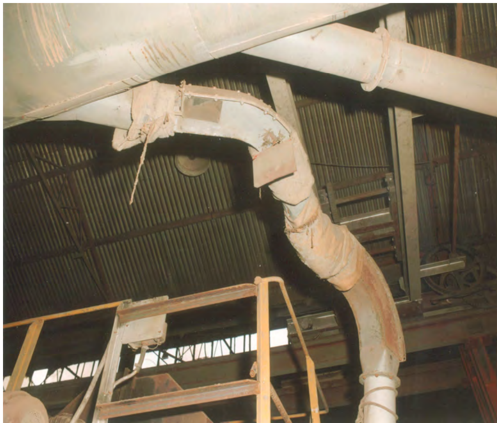
Figure 35: Makeshift repairs to the ducts with hessian sacks. Photo
