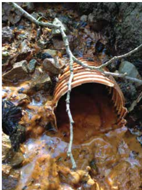
Figure 11. Drain jetter and blockage due to iron ochre
