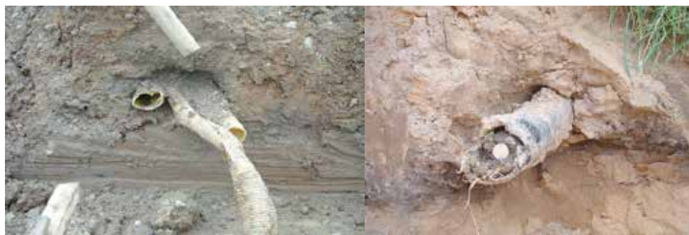
Figure 10. Examples of old and blocked pipes
