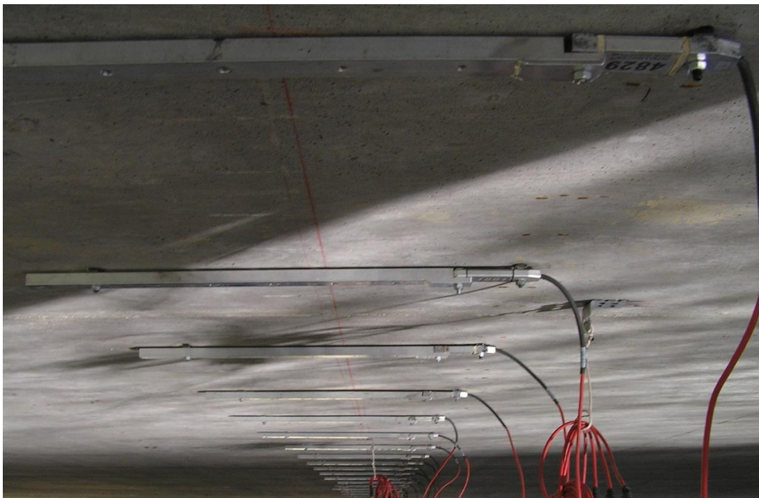
Figure 8. Johnson County Bridge strain transducer
