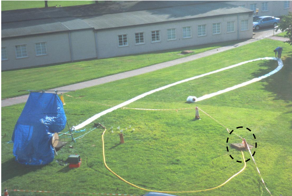
Figure 5.6: Picture of the test site with the “Bigsock” before the installation in BH1. The dotted ring encloses the sewer cover used for discharge.
