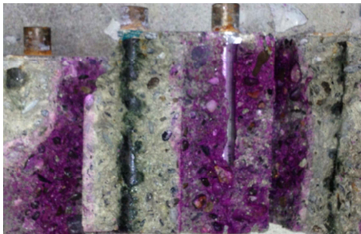
Figure 4-18 Sample 4C-30 after autopsy, on the active bar corrosion products are only formed at steel concrete interface
