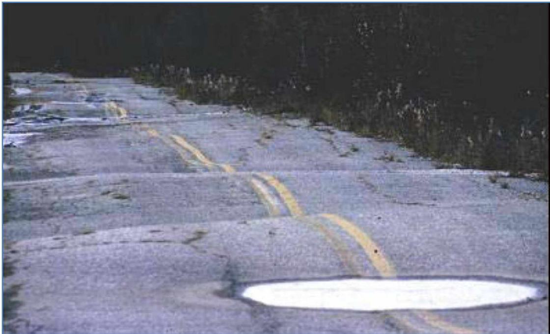
Figure: 1.4: Waviness in roadway embankment due to thawing permafrost
