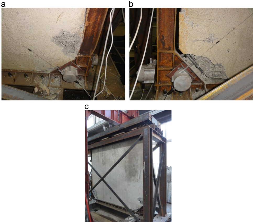
Fig. 10. Lower corners of the Configuration 1 SRCW specimen after the failure: a) shear failure of the non-dissipative zone, b) spalling of the concrete and complete detachment by the steel frame and c) global view.
