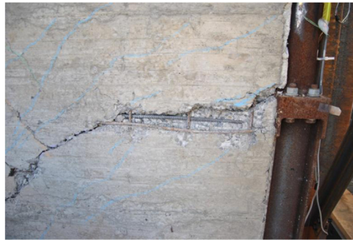
Fig. 15. Failure of the reinforcing bars crossing the main crack.
