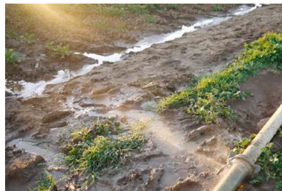
Figure 9 Leakage in pipe
