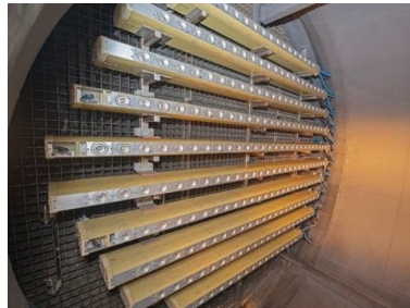
Water injection spray bars installed in PSL test cell
