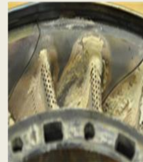
Typical build-up on vane
