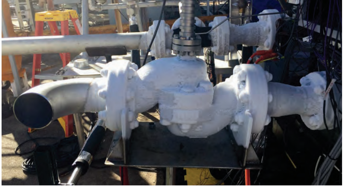
FIGURE 2. A facility cryogenic vent in use during IVF testing.
