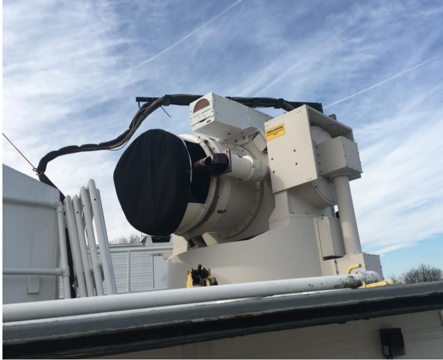
Figure 2. The piggybacked beacon telescope-fiber optics assembly on top of the NASA SLR telescope at the MOBLAS facility.
