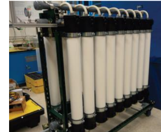
The Water Recycling System
