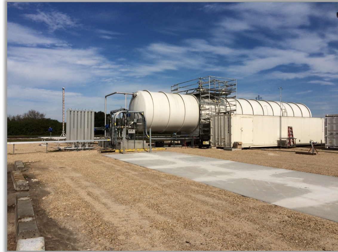
Ground Operations Demonstration Unit for Liquid Hydrogen (GODU-LH2)
