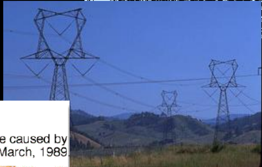
PJM Public Service Step Up Transformer
