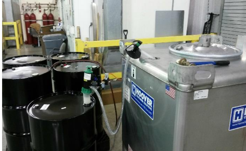
Figure 15: Novec™ HFE-7100 barrel to 350-gal SS tote [14] transfer operations.
