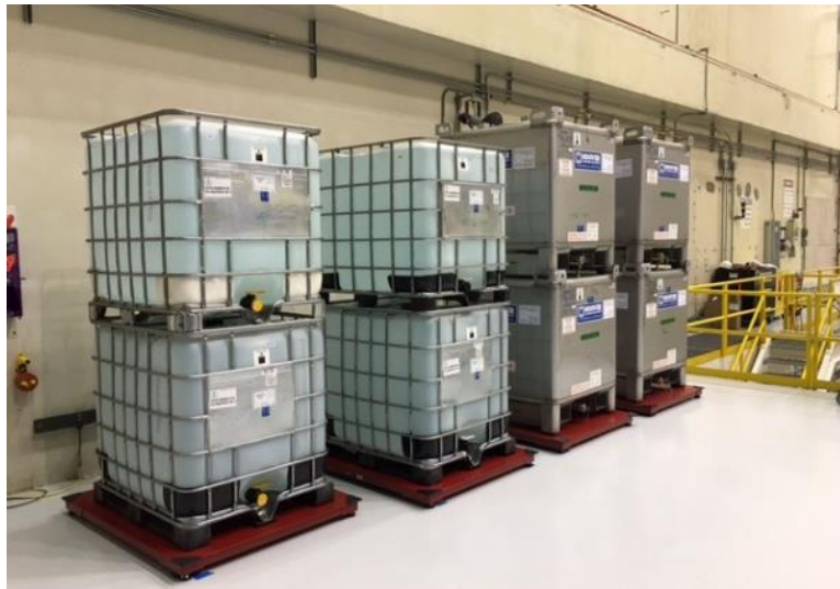
Figure 17: Deionized (DI) water and Novec™ HFE-7100 storage totes [9], [14] on weight scales [16].
