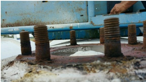
Major corrosion on studs
