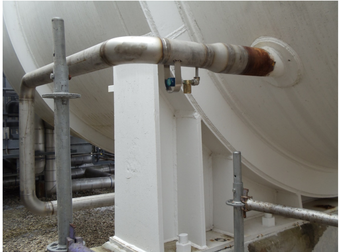
NEW INSTALLED VACUUM PIPING
