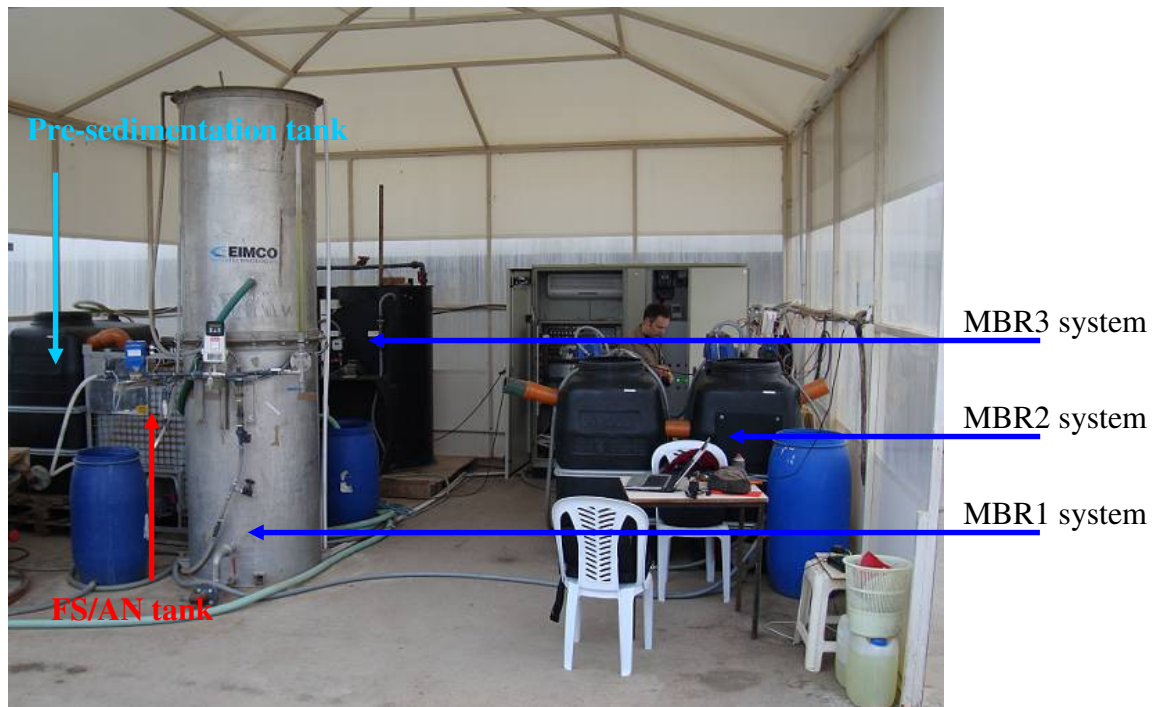
Figure 3.16 The MBR pilot plant installation
