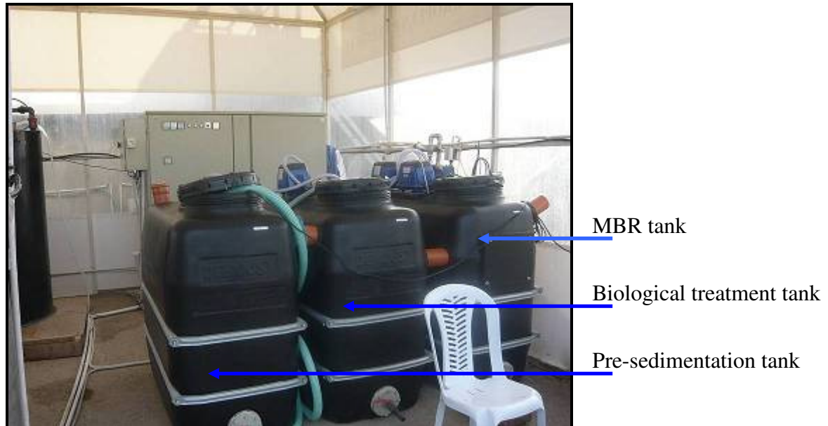
Figure 3.8 The MBR2 system - The control panel is in the cabinet in the back
