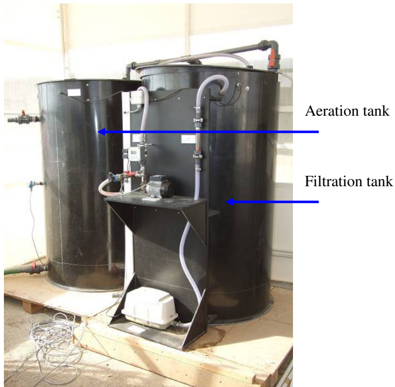
Figure 3.12 The MBR3 system - The control panel is shown in Figure 3.7
