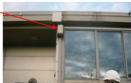
(12) RFID reader fixed on the gate
