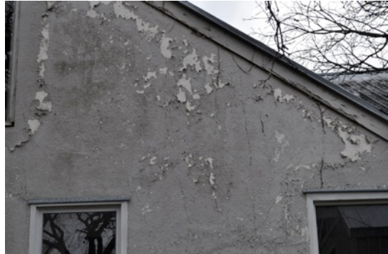
Moore/Andersson paint deterioration detail
