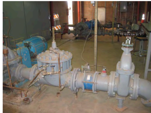
View of pump station for water reservoir.
