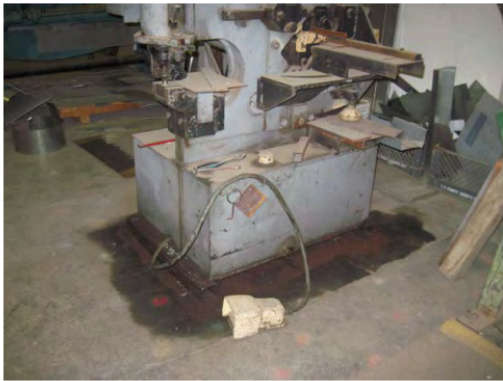
Hydraulic oil beneath hole punch machine in George Barracks.
