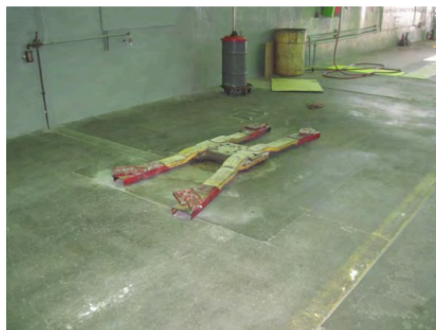
View of apparent hydraulic hoist in Vehicle Fleet Services Garage.
