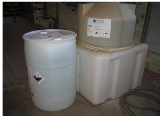
View of corrosion inhibitors and chemicals used at Steam Plant.
