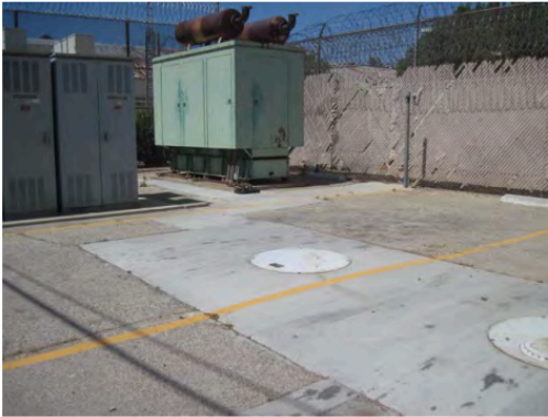
View of emergency generator and 4,000-gallon diesel fuel UST north of Bldg. 3.
