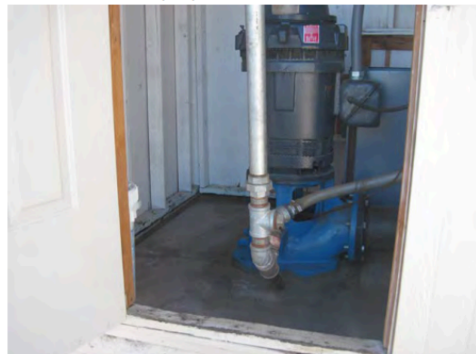
View of Well #3 water pump station.
