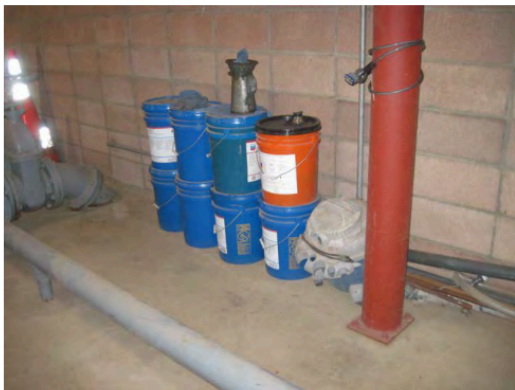
View of 5-gallon containers of oil stored at pump station.
