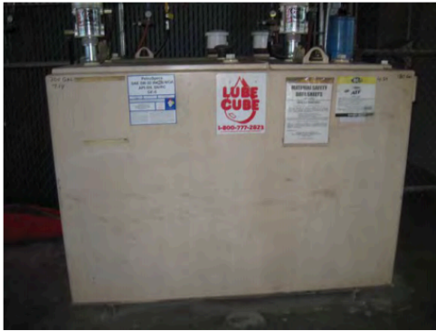
300-gallon new oil/100-gallon transmission oil in Vehicle Fleet Services Garage.
