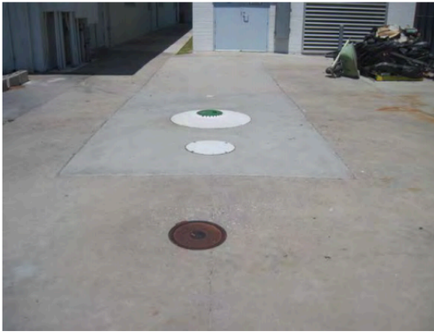
View of 4,000-gallon diesel fuel UST for Hospital emergency generator.
