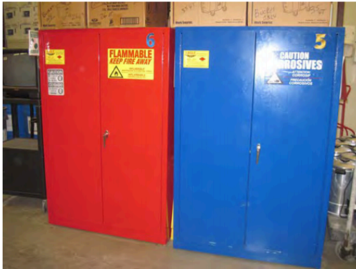
Flammable/corrosive cabinets seen throughout the facility. These in Bldg. 5.
