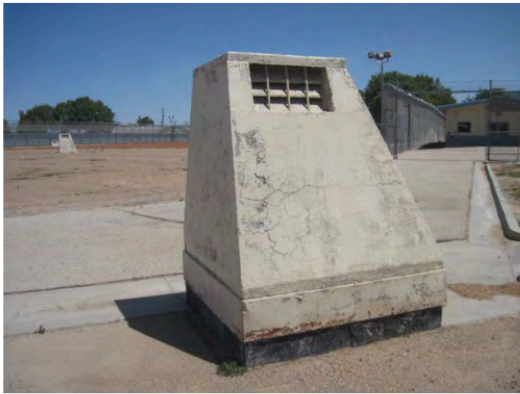
View of steam tunnel access and vent at Mira Loma Detention Facility.
