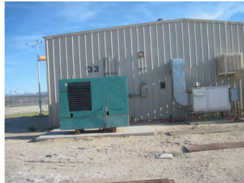
View of emergency generator at Building 33.
