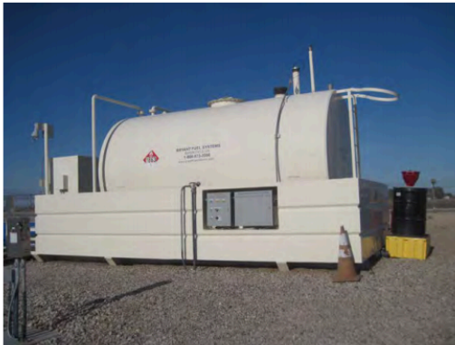
View of 5,000-gallon jet fuel AST at Heliport.
