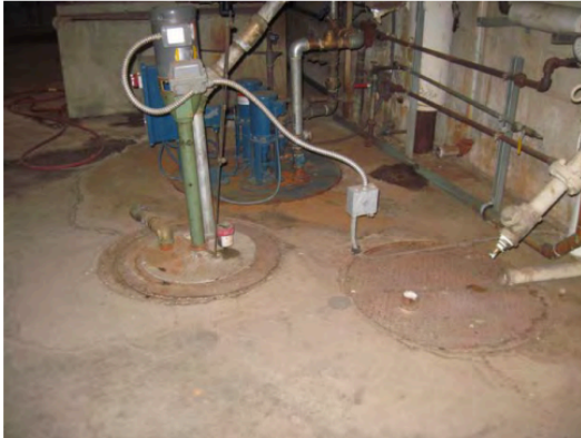
Sumps located in Building 4165 (Kitchen) basement.
