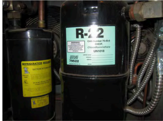
Refrigerant for large commercial refrigerators in Building 4165.
