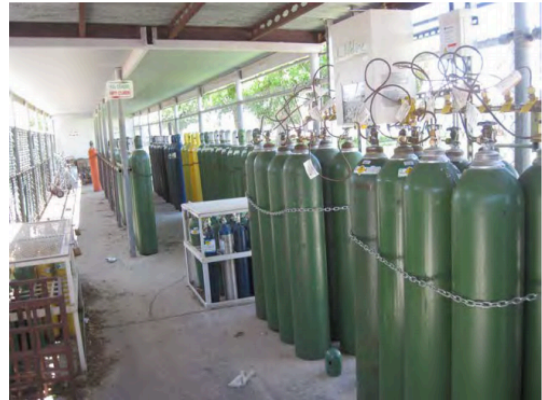
View of nitrous oxide and oxygen cylinder storage outside Hospital.
