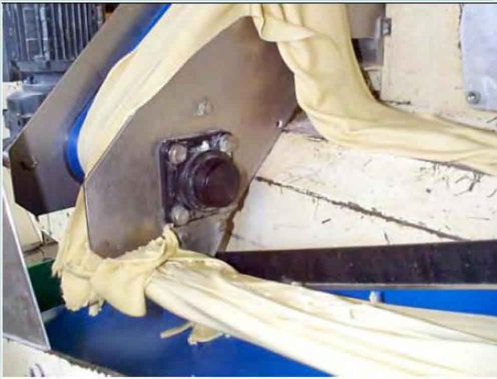
Bearing as high risk lubrication point
