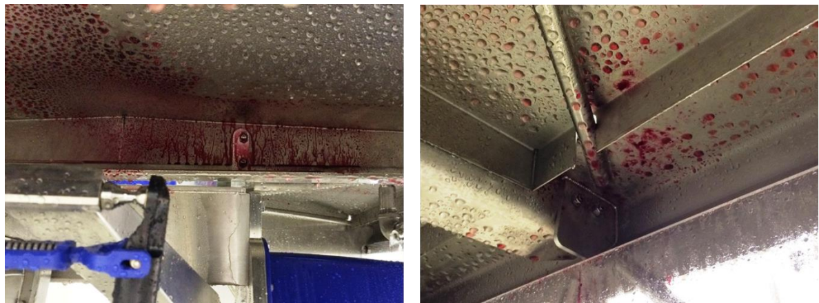
Fig. 50: Delta Robot after extra 10 minutes of cleaning with the full cone nozzles – spray shadows.
