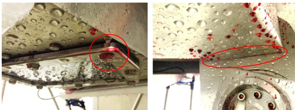
Fig. 45: Delta Robot after 10 minutes of cleaning with the fixed nozzles – crevices, metal-to-metal-connections.
