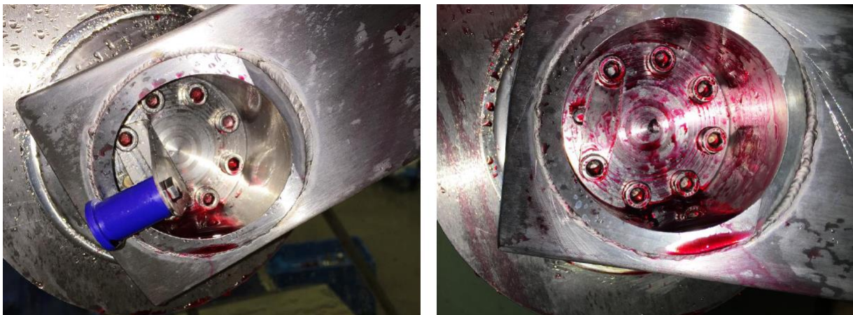
Fig. 64: Not cleanable and drainable areas inside the orifices at the motor blocks.
