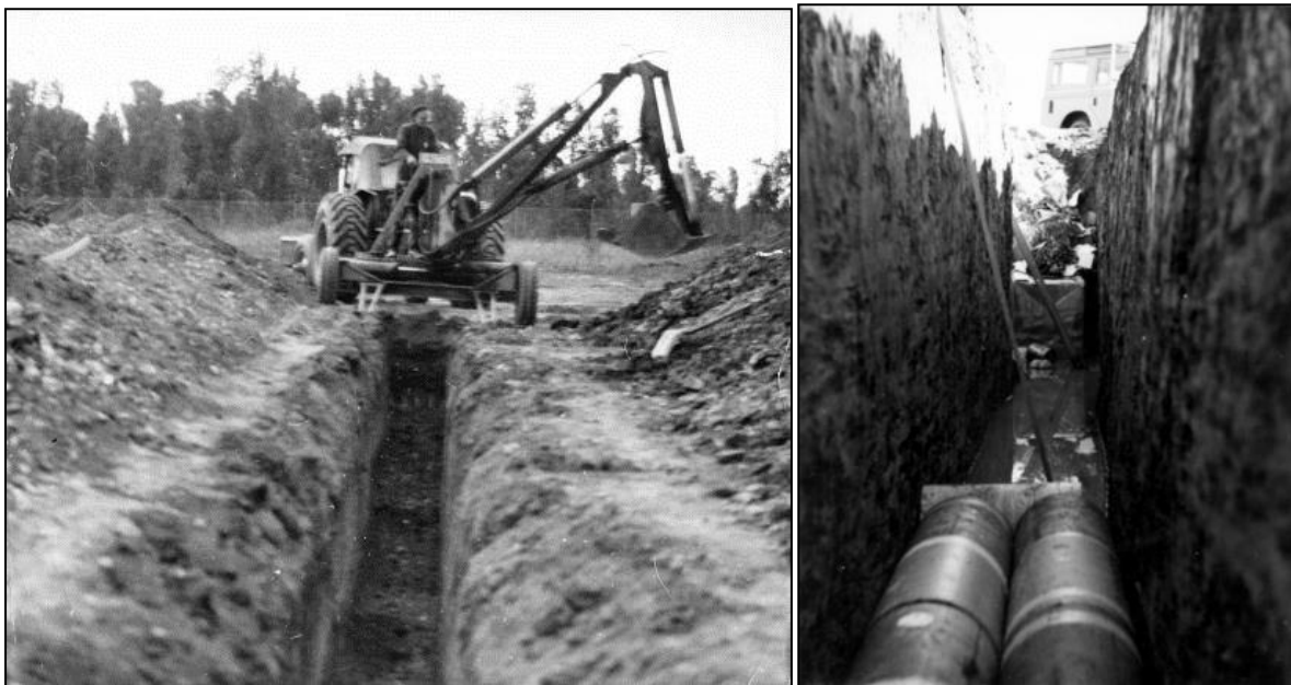
Figure 3. Contemporary photographs of (a) trench excavation and (b) trench disposals. In (b) the presence of a significant amount of water is visible beyond the drums in the foreground [this is more obvious in the original print].
