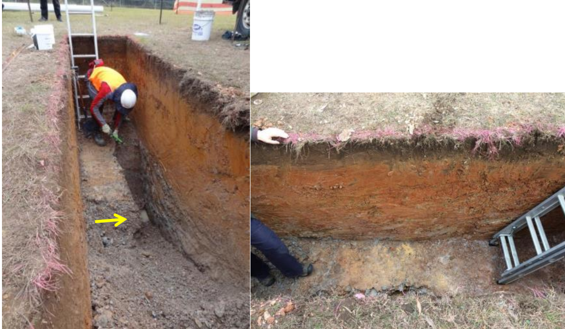
Figure 51 (a) Photographs of a small amount of seepage observed from shallow layers (b) View of southern edge of trench after initial excavation (to ~1.2 m).
