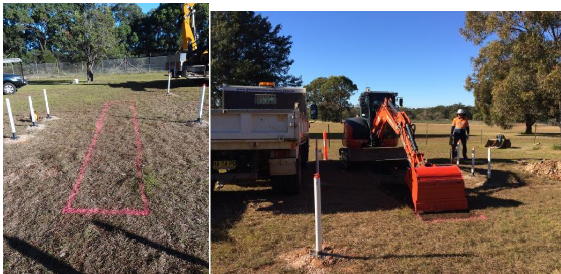
Figure 26. (a) Marking out the area for the pilot trench. (b) commencement of excavation (Monday 26 th June).
