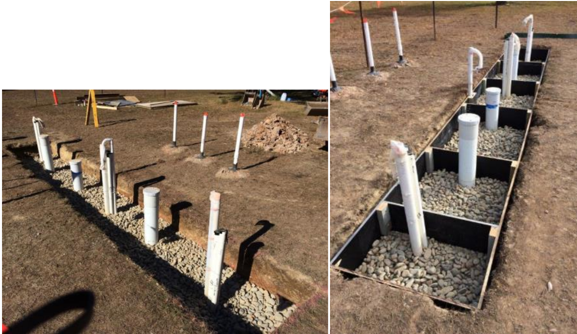
Figure 34. (a) Final state of the trench after filling with pebbles to within approximately 300 mm of ground surface (b) After installation of plywood to protect the side walls of the trench. Following extensive discussion it was decided not to cover the pebbles with a soil layer as this would have introduced a flux of particles into the pebbles which would have progressively affected hydraulic properties. The option remains to install a soil cover at a later date if desired.
