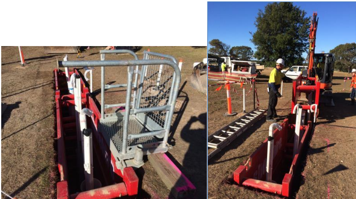
Figure 31. (a) Installation of the sampling tubes and in-trench piezometers (Friday, 30 th June, 2 pm). (b) Removal of shoring boxes (Friday 30 th June, 3 pm). The removal of the shoring boxes was a delicate operation, with special care being taken to avoid disturbing installed piezometers.
