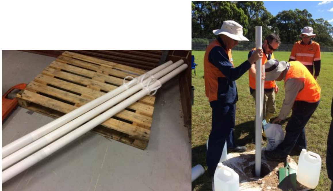
Figure 19. (a) Pre-constructed piezometer, note the slotted section and spacers to keep it central in the hole. (b) Installation of sand-pack around slotted section. For more details, see Figure 25.
