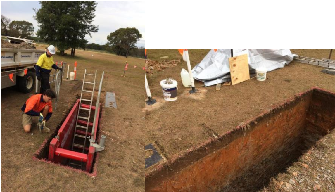
Figure 29. (a) First installation of a trench shoring box in the partially excavated trench (Tuesday 27 th June, 3 pm). (b) Photograph of trench with shoring box removed (Wed 28 th June, 1 pm).
