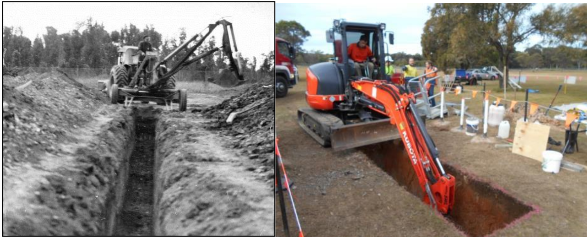
Figure 62. Comparison of photographs of (a) excavation of historic trenches and (b) of the pilot trench.
