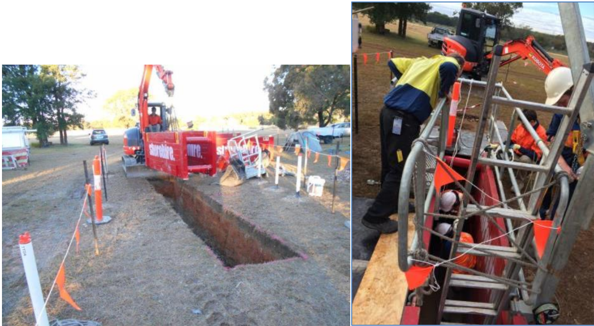
Figure 30. (a) Installation of a shoring box in the completed trench (Thursday afternoon, 29 th June). (b) In-situ inspections of completed trench within shoring box (Friday 30 th June, 10 a.m.).
