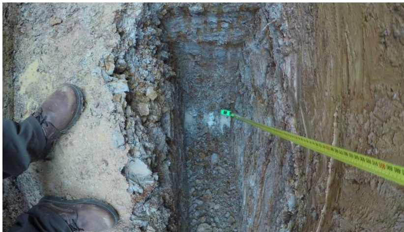
Figure 54. Seepage into Pilot Trench below the hard shale/siltstone layer at ~2.15m depth
