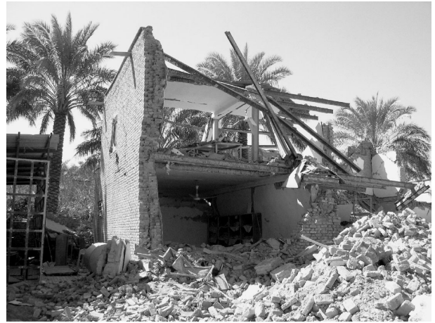
Photo 6. Collapsed two-story school building.
