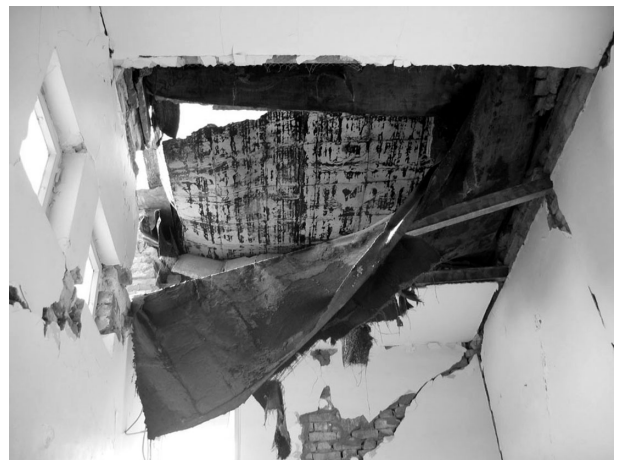
Photo 4. Falling down of the roof of penthouse.
