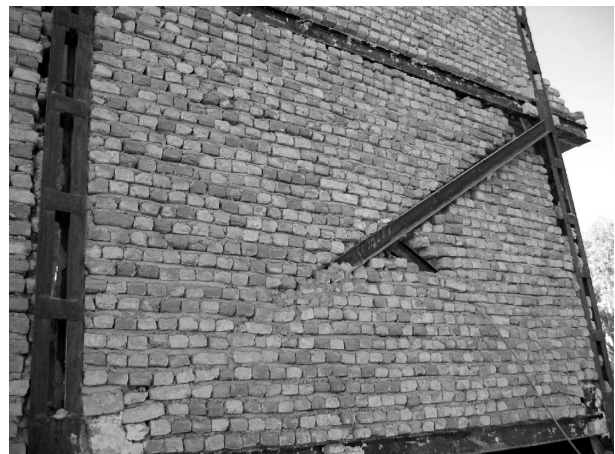
Photo 10. Buckling of steel brace and damage to brick wall.
