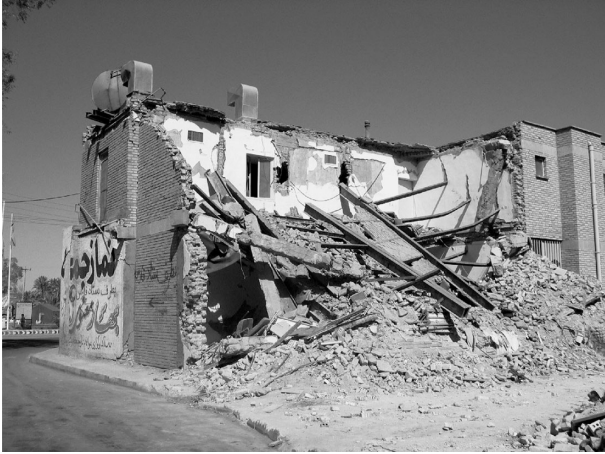
Photo 2. Collapse at the south west section.
