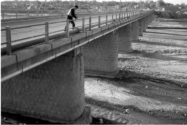
Photo 9. Appearance of Esfikan bridge after the earthquake.
