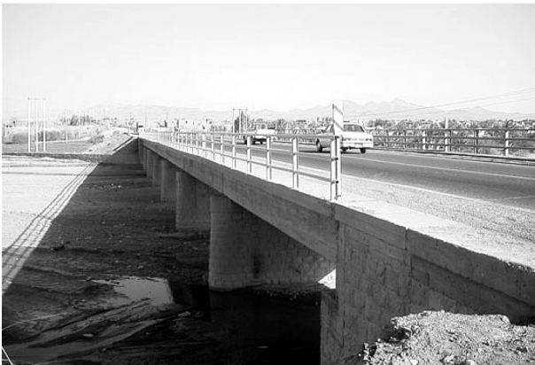
Photo 10. Appearance of Khaje-Askar bridge after the earthquake.
