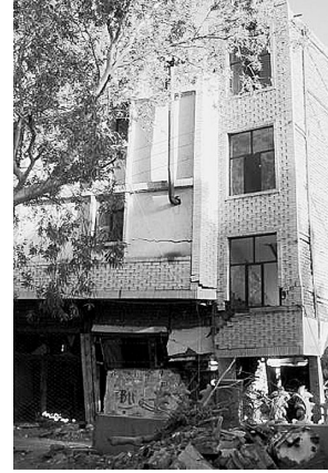
Photo 15. Damaged building in front of bank in Photo 13.
