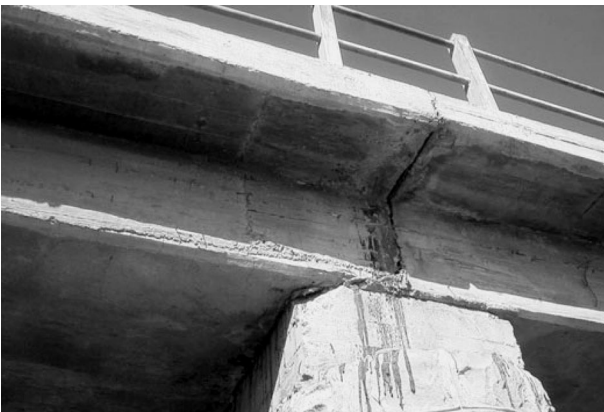
Photo 11. Minor displacement of Esfikan bridge at the top of pier.
