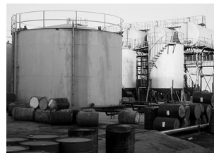
(a) Tank and pipes.
