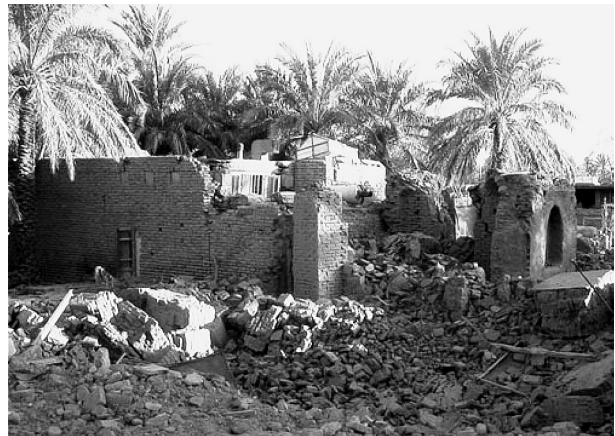
Photo 16. Foundation of destroyed adobe house.
