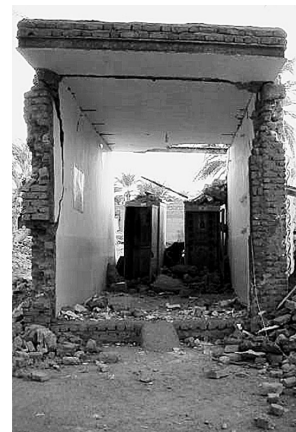
Photo 17. Damage of to masonry structure.
