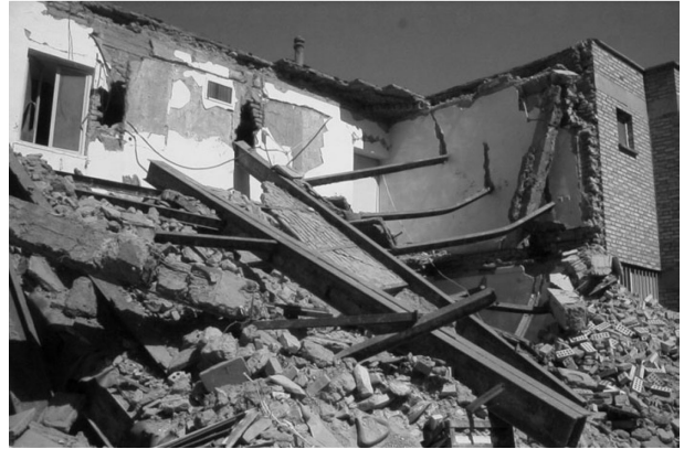
Photo 4. Damaged masonry building near site of IIEES array 6.
