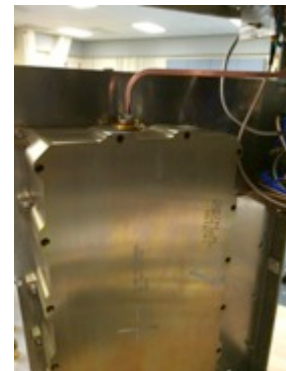
SSPA installed in CRS
