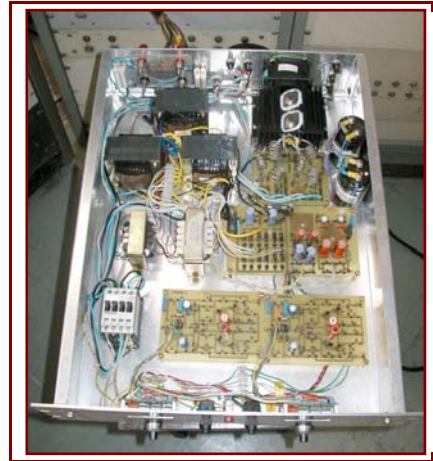
Figure 1. Current power supplies top view.
